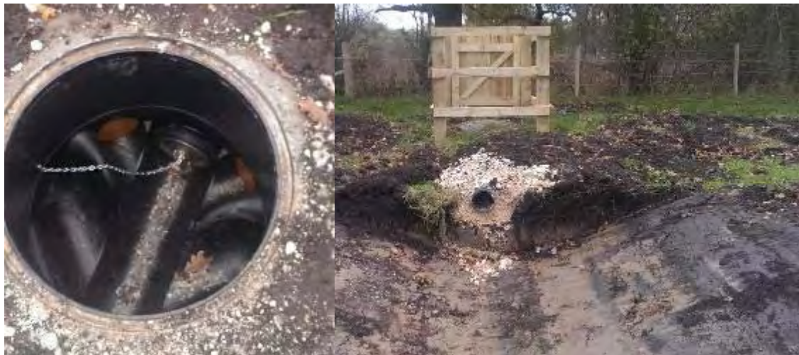
Figure 6-7: Example of a water distribution gateway to control the flow of water between individual scrapes.
