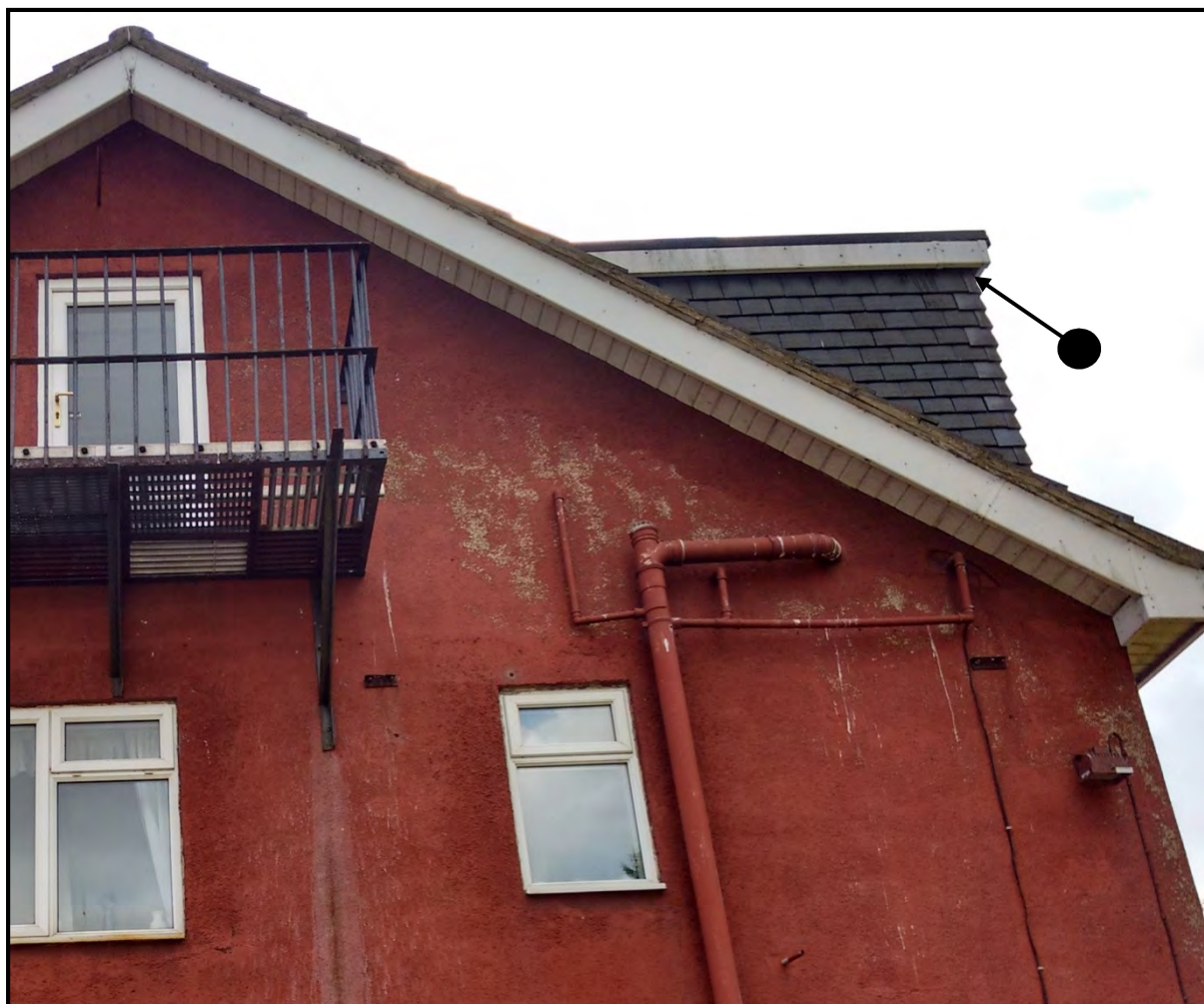
Plate 1: View of east elevation of main residential property at Hazel Dene showing the location of access by common pipistrelle during the dawn swarming survey of 22 July 2016 (indicated by arrow).
