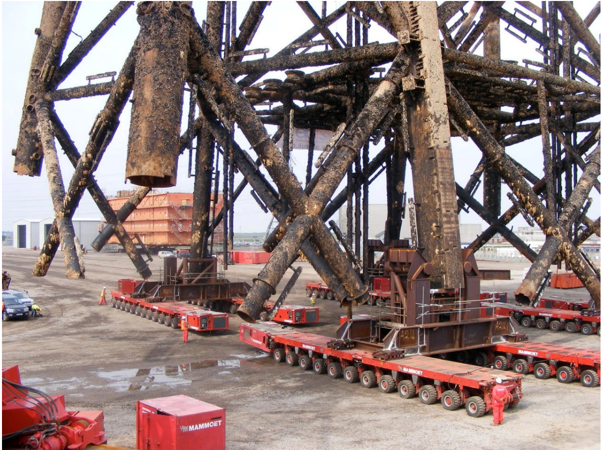
Plate 3 : 1500 Tonne section of North West Hutton Jacket being moved by SPMT on a stone surface at Able Seaton Port. (Note the large expanse of flat site)
