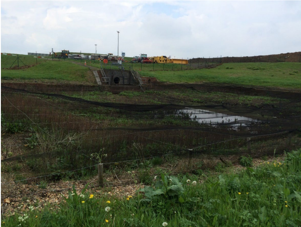
Photograph 25: Pond 15 – Drainage infrastructure forms part of SUDs associated with runway infrastructure (2018).
