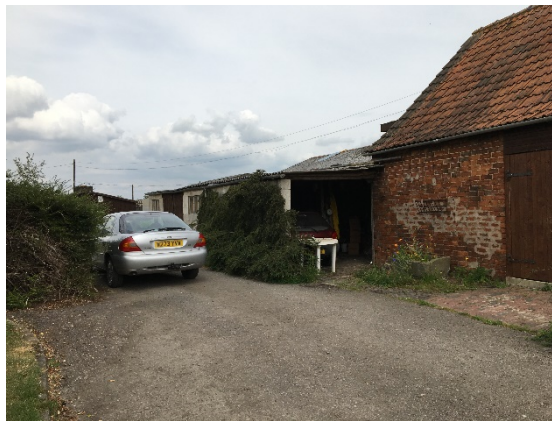
Photo 2-2 BU_378 external showing lean to with access points in the brick work to the cool room.
