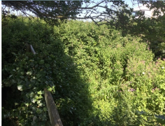
Photo 13 (2019): Leigh Brook Culvert could not be seen upstream of the Leigh Brook Culvert due to overgrown vegetation. No perceptible flow at this location at the time of survey.
