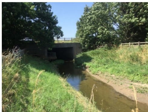
Photo 7 (2019): View of River Chelt Culvert inlet, with deposition collecting on the right bank. An artificial embankment was also present along this stretch.
