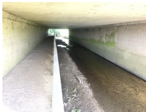
Photo 8 (2019): View through the River Chelt Culvert showing fine sediment deposition. Trash and vegetation which were assumed to be flood deposits observed on the concrete walkway indicates flows have been much higher within this reach.
