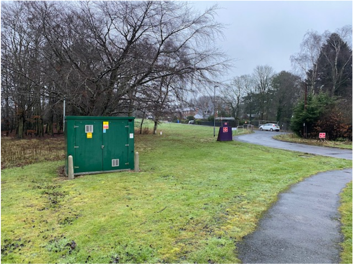
Gas house at southern end of West View well away from existing houses and road
