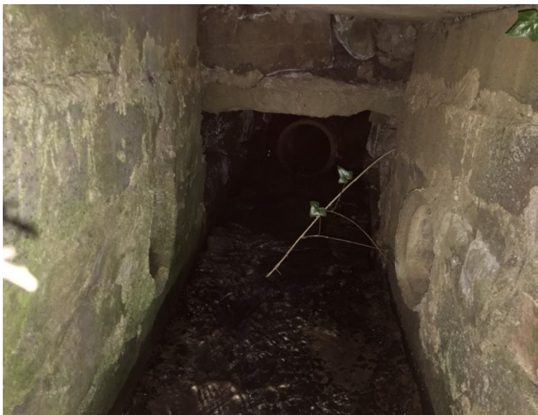
Figure 5-4 – Farm Access Track Culvert along Tributary of White House Burn (Outlet)
