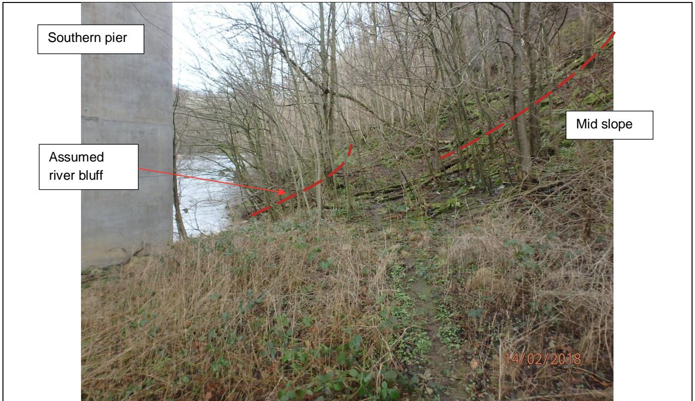
Photograph 3 – View east from the position of the southern pier of the existing A1 bridge. Note the reducing gradient of the midslope (possible colluvium) and the river cut terrace.
