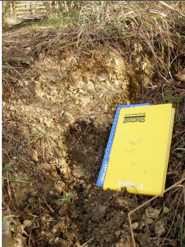
Photograph 14 – Made Ground materials described within tension crack 3 adjacent to the footpath steps. The major divisions on the blue card are 1cm wide. The thickness of the upper unit is approximately 20cm.
