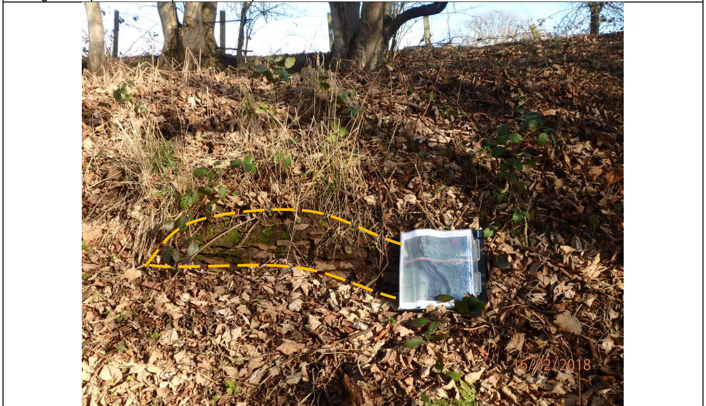
Photograph 17 – Exposed corrugated metal sheets, below the level of the footpath, exposed within the backscarp of one of the failed blocks. Photograph taken at NZ 17545 99955. Clipboard is A3 sized.
