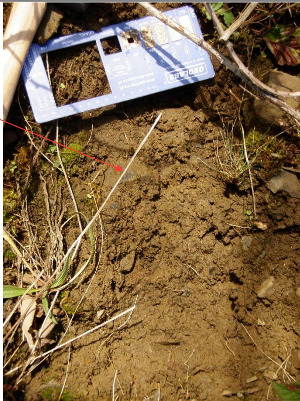
Photograph 15 – Detail of the lower Made Ground as seen within the scarp of tension crack 3.
