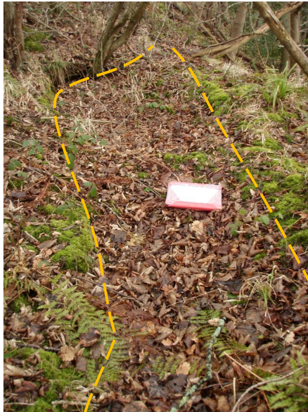
Photograph 12 – View east of a tension crack within a failed block. This structure is located to the south of the public footpath. The clipboard within the photograph is A4 sized.
