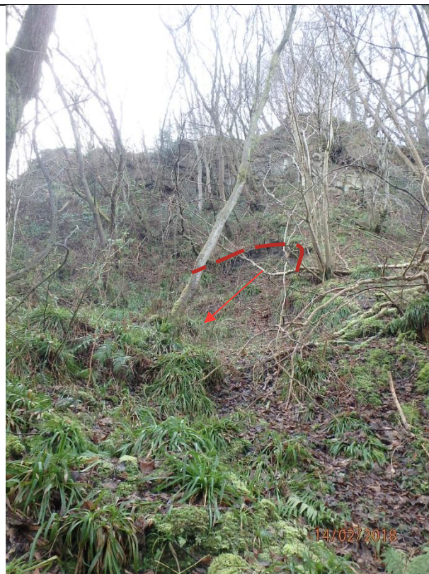
Photograph 10 – Arcuate scarp noted to the west of the southern embankment. This feature appeared to be fairly recent, with exposed soil within the back scarp.
