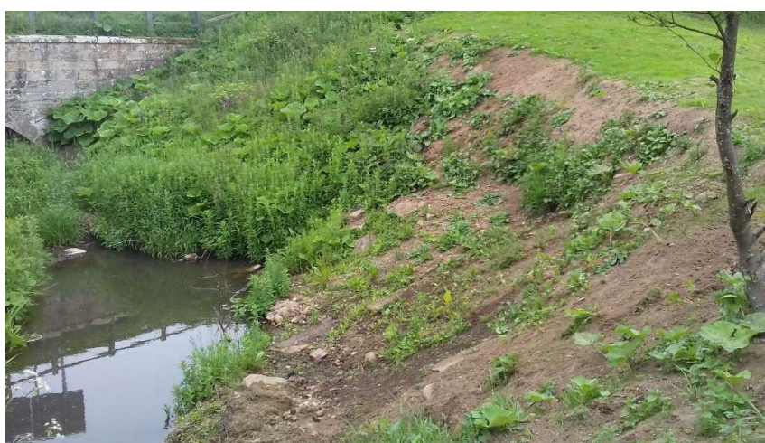
Figure 10-3 – Evidence of Erosion along Longdike Burn
