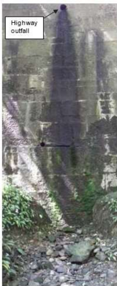
Figure 7-3 – Evidence of Erosion Underneath Outfall
