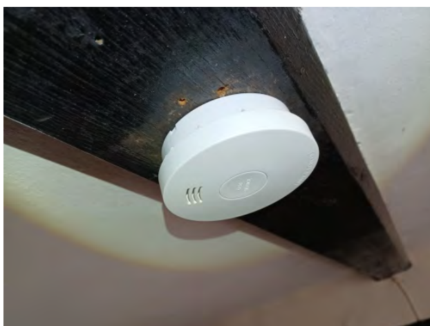
Fig.22: Smoke detector located within the ground floor lounge.
