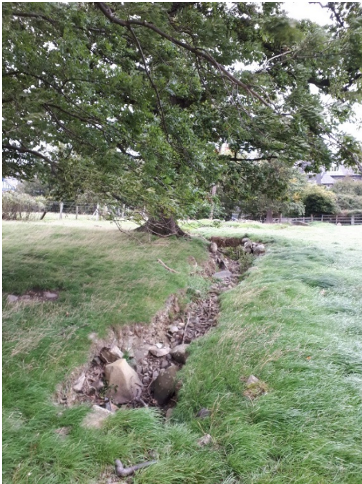
Plate 3 – Scoured Channel near Penmaen Park
