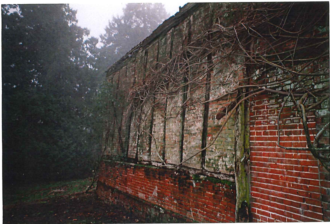
The east elevation of range G showing the timber framing and brick panels
