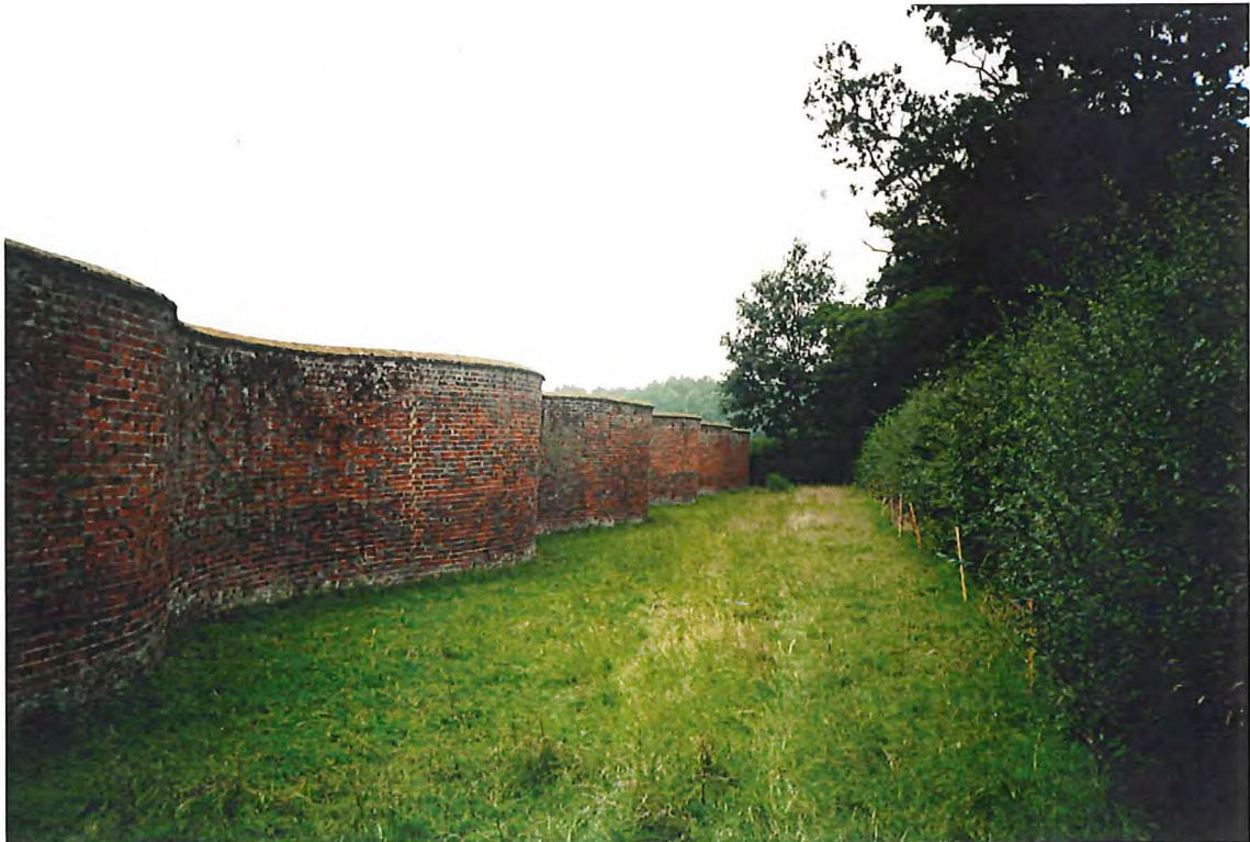
The north wall of the kitchen garden seen from the north east
