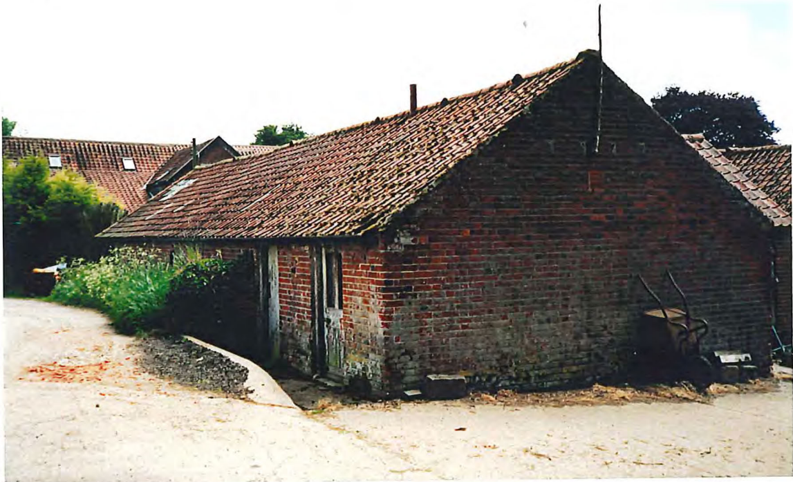
The north and west elevations of range B seen from the north west
