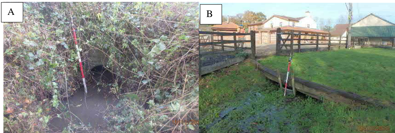
Figure 5-4 (A) Inlet and (B) outlet from the culvert downstream of the A47
