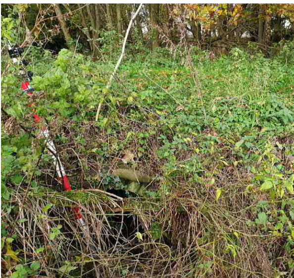
Figure 5-7 Inlet to culvert 11 showing significant blockage
