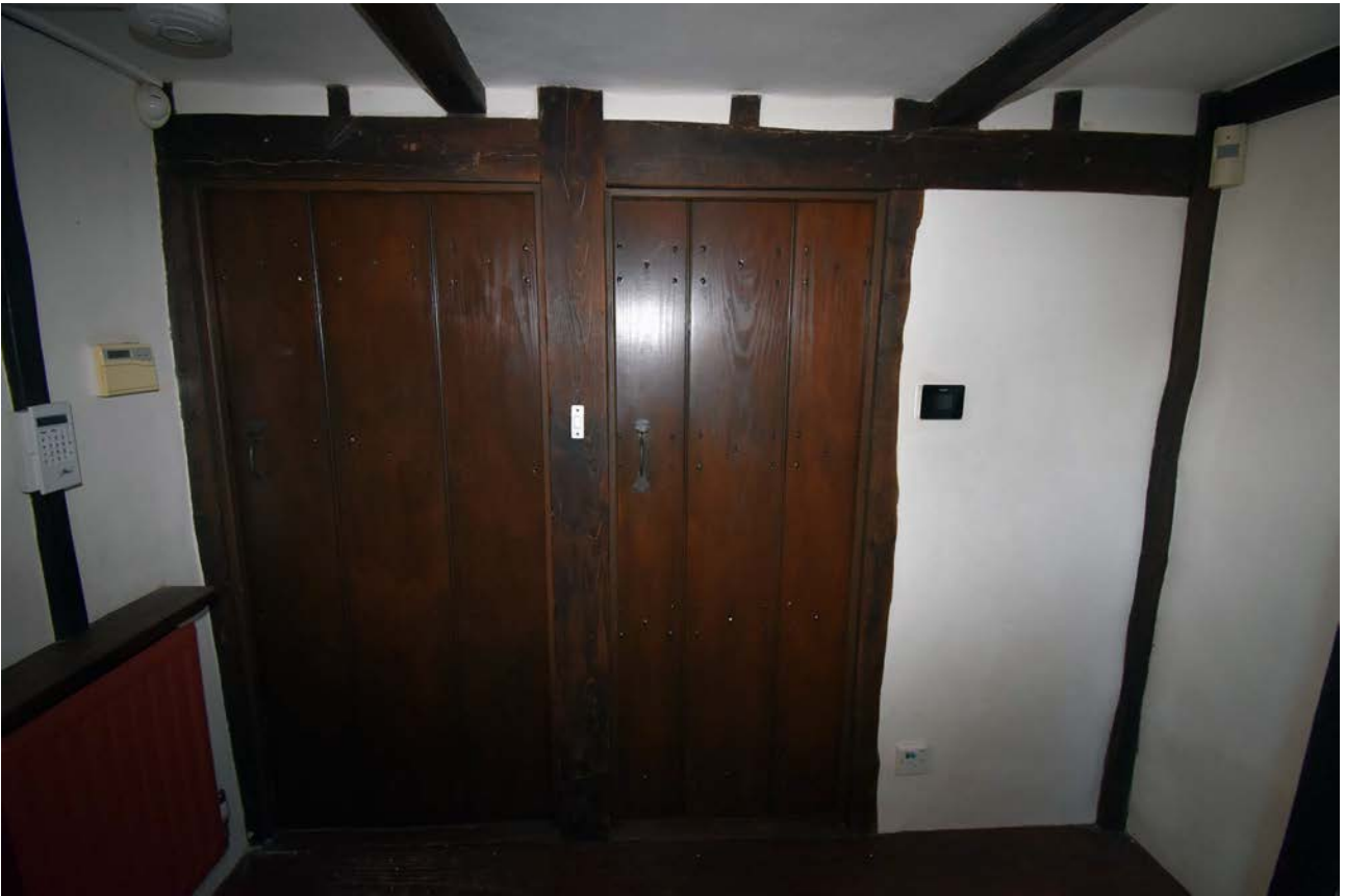
Plate 55: Ground floor, entrance hall, south wall, close doors to lobby and bathroom
