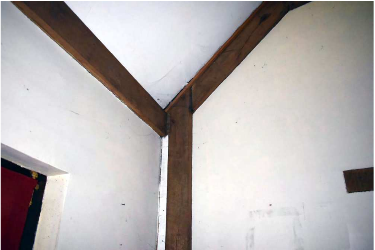
Plate 95: Extension, north bay, north- east corner, join of the principal rafter with the post and ceiling beam
