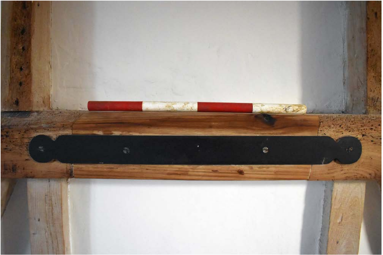
Plate 90: First floor, principal bedroom, east wall, iron strap with piece of modern inserted
