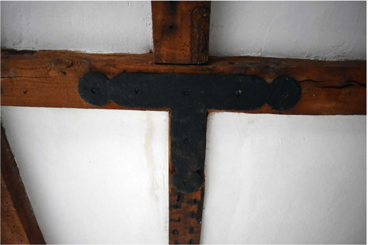
Plate 74: Ground floor, living room, south- east corner of ceiling, trimmer joist with an iron strap T-shape
