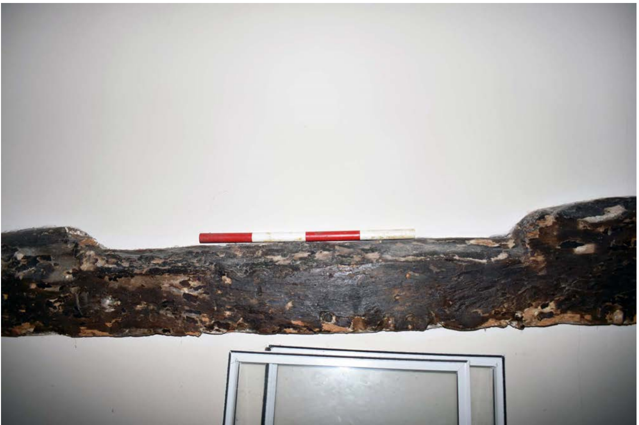
Plate 24: Indent on the tie beam of principal bedroom in The Thatches
