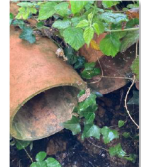
Second visit on 31 May 2022, no flow, only seepage underneath the pipes
