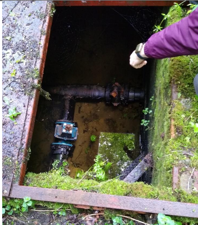
Photo ref. 1 – Direction north. Pea Lane and M25 – adjacent headwall. Pipework beneath manhole cover related to irrigation system that takes water by gravity to a reservoir in the west and can also act in reverse to pump water back east to supply abstraction points to the east of the M25.
