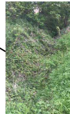
Heavily vegetated. Some mildly flowing water observed
