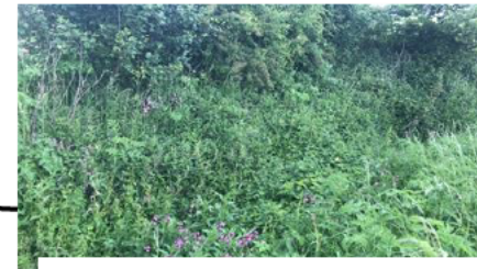
Too vegetated to observe water. Pipe completely obscured. No audible water flow 24 May 2022
