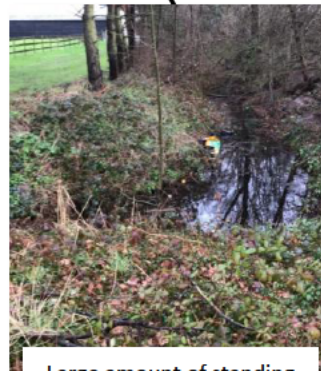
Large amount of standing water but no flow
