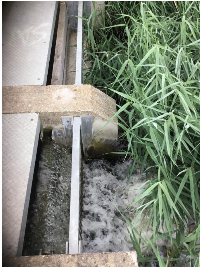
SY-1S05ZZZ5– Shorne Marshes, surface discharge from the northern part of the Ramsar (Denton New Cut) into the Thames and Medway Canal
