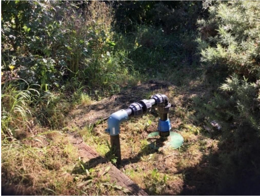
GD-2S05ZZZ1– Abstraction borehole, located along the track to the course, between the green keeper shed and the reception.
