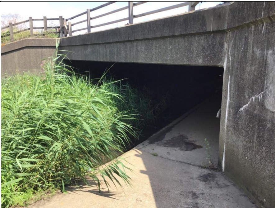
SN-1N17ZZZ1– Culvert of the West Mardyke below the M25 and adjacent to the Thames Chase Forest Centre
