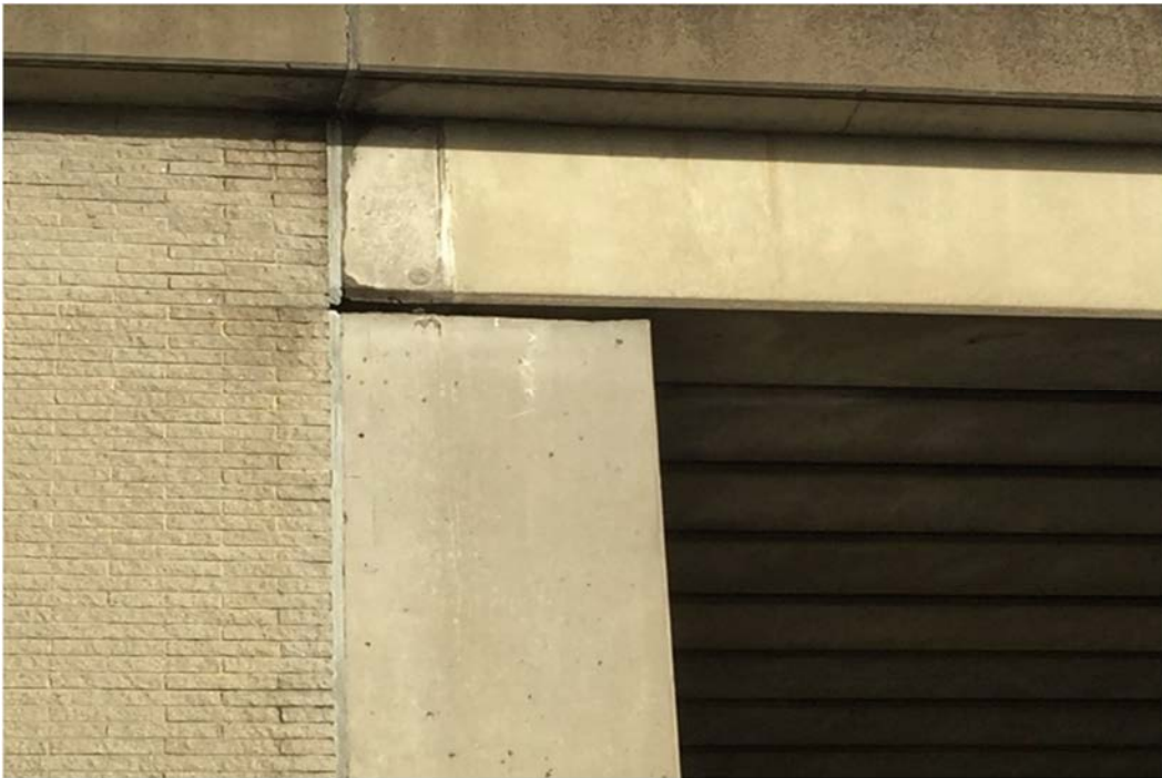
Photo 7- Potential roosting feature of the gap between the abutment and bridge deck on the north-east side of Eighton Lodge north Underbridge
