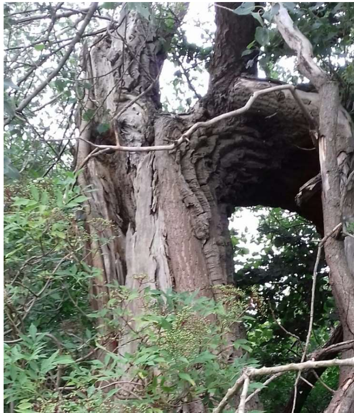
Photo 20 – Large cavity/hollow in trunk of Tree T3, likely as a result of a tear out.
