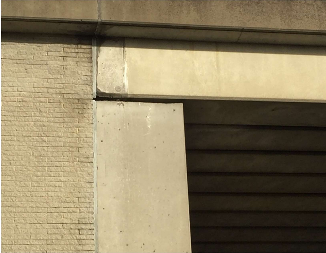
Photo 7- Potential roosting feature of the gap between the abutment and bridge deck on the north-east side of Eighton Lodge north underbridge
