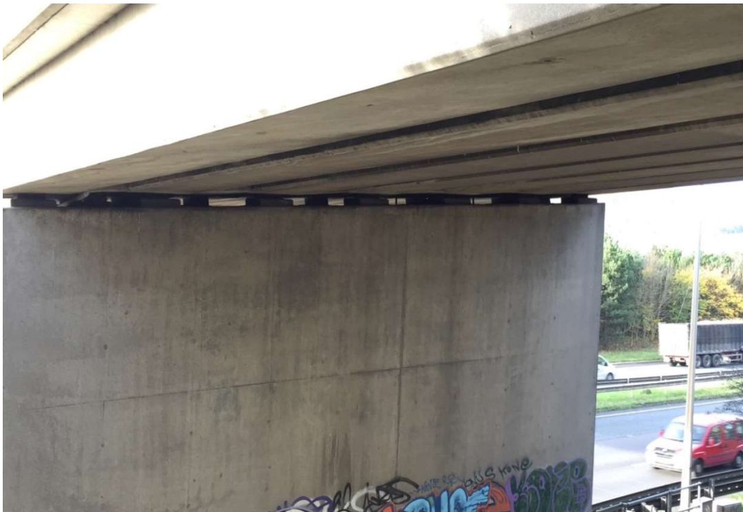
Photo 2- Potential roosting feature of the gaps between abutments and bridge deck on Smithy Lane Overbridge, as well as the gaps between the concrete beams on the underside of the bridge deck
