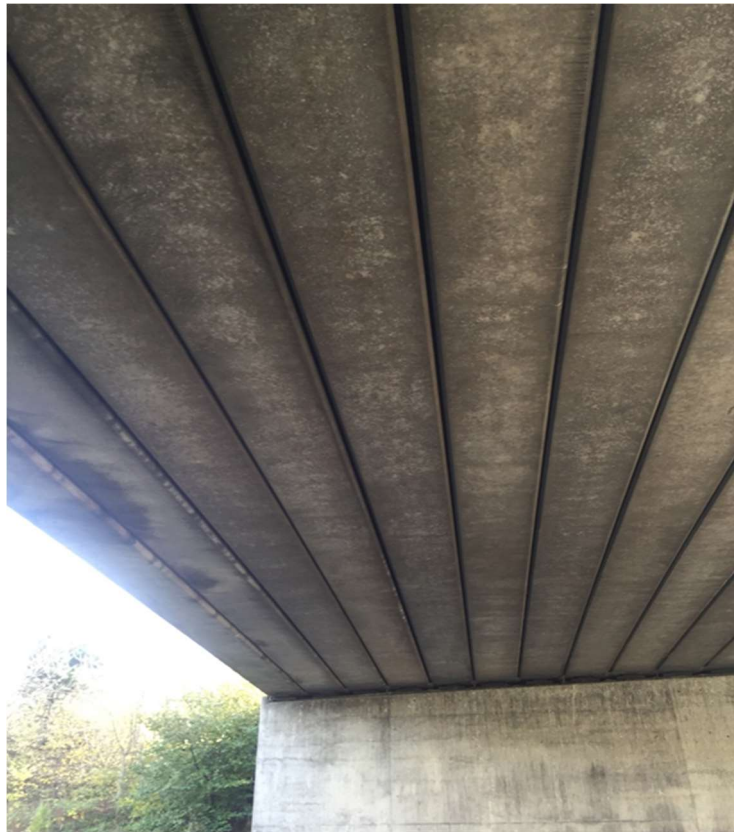
Photo 8- Potential roosting feature of the gaps between the concrete beams on the underside of the deck of Eighton Lodge north underbridge
