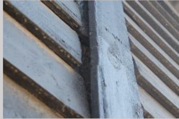
Photograph 2: Gaps under the shiplap boarding within Building 1.
