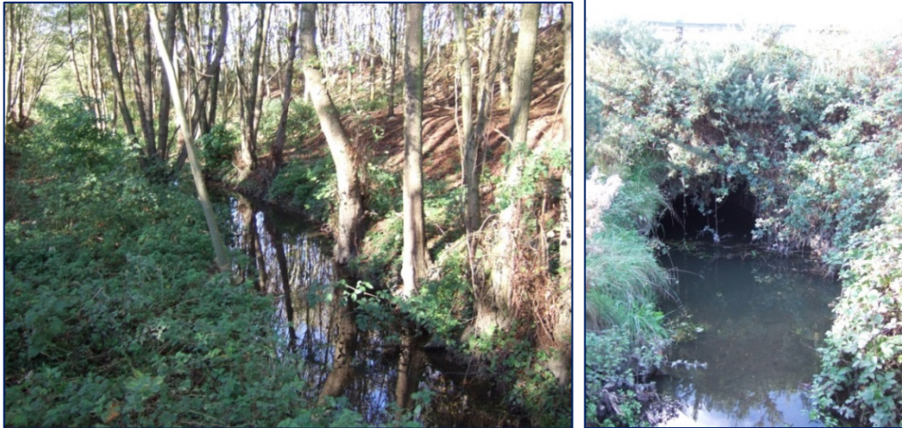
Photo 1a (left) Hollywell Brook just upstream of the M42 culvert; Photo 1b (right) Hollywell Brook downstream of the M42 culvert.
