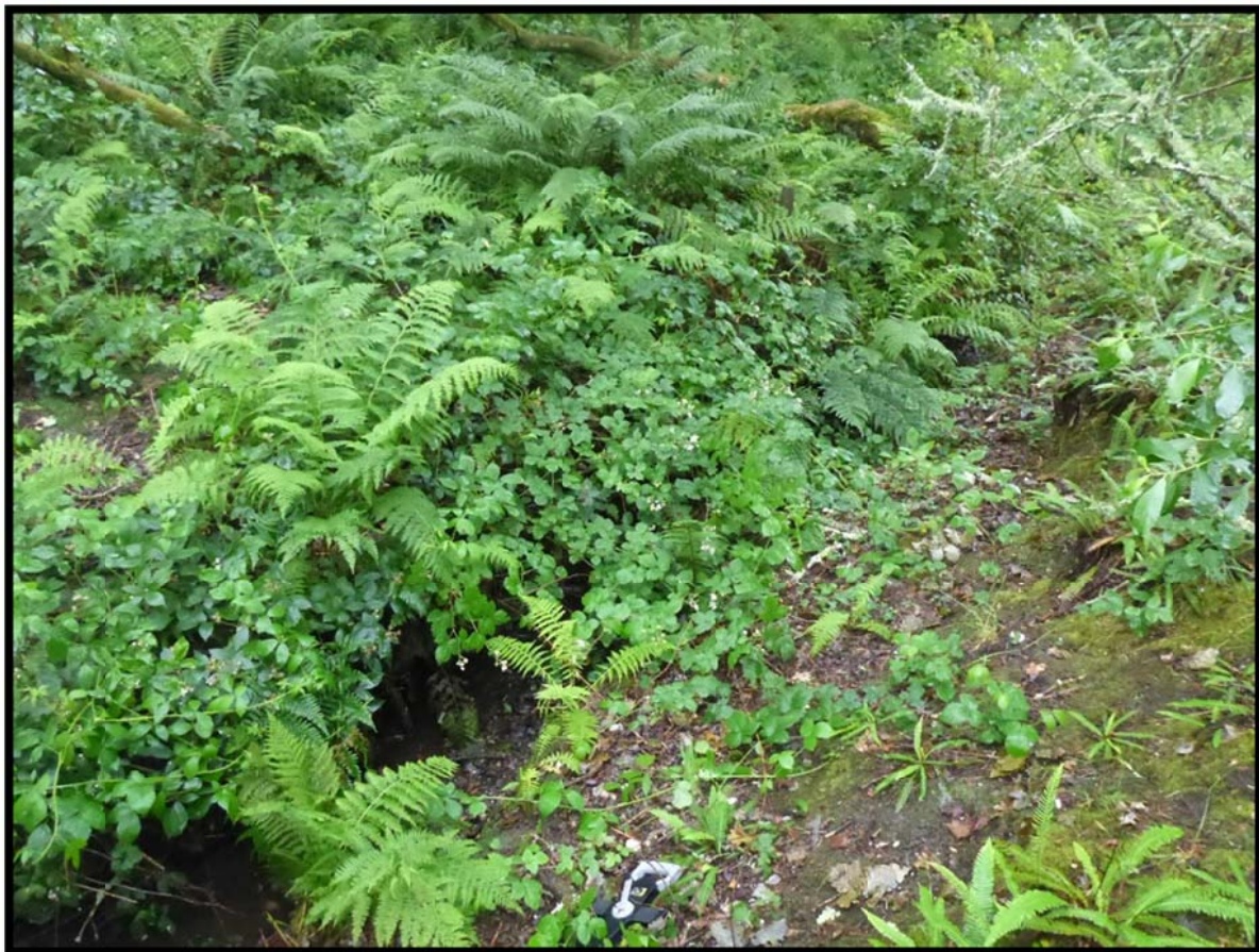
Figure 3 Overgrown channel at Site 5.2
