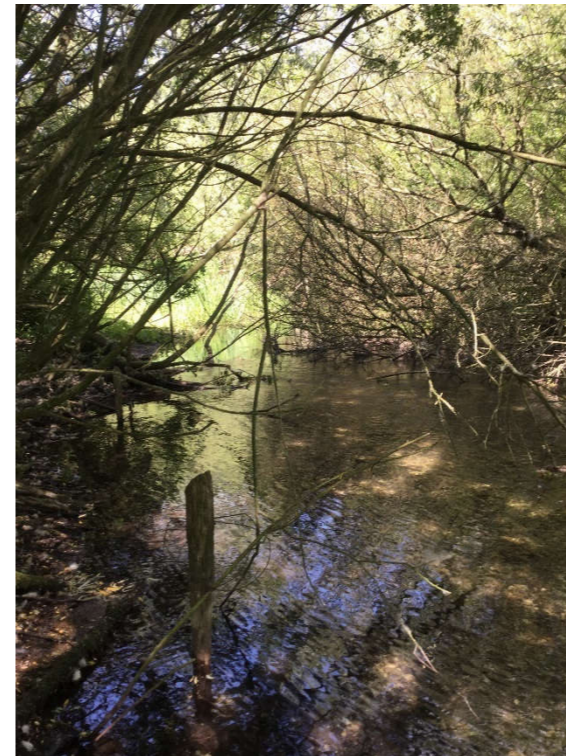
Photo IMG_0040: Defunct deflectors/historic reinforcement
