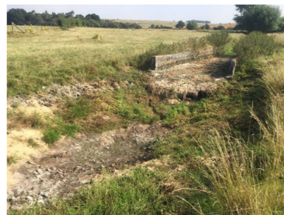
Photo ATT-65 – Scour downstream of structure
