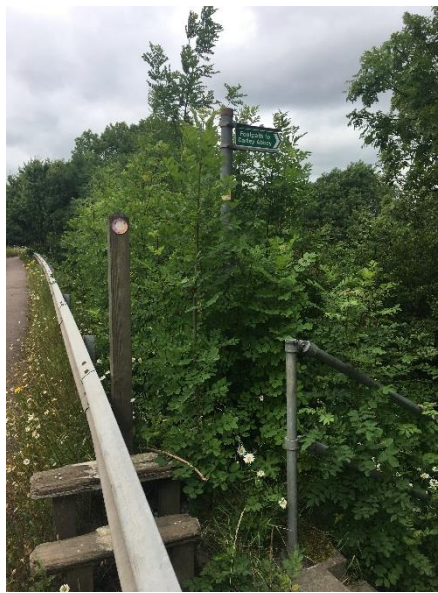
20: Safety barrier across the entrance of Breadsall footpath 7
