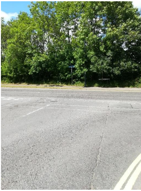
37: Poor sign visibility for NCN 54, 68 + RCR 66
