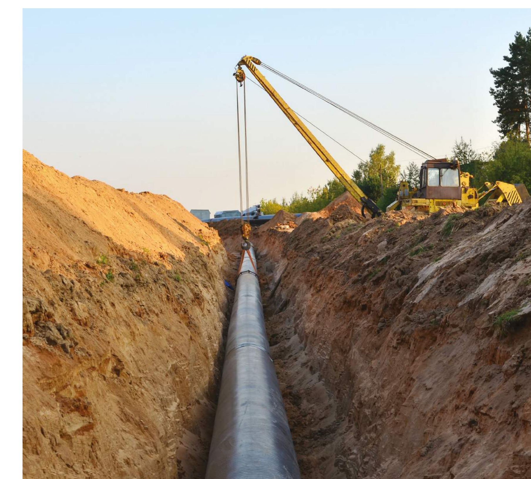
The CO 2 will travel from Immingham through a new onshore pipeline to the former Theddlethorpe Gas Terminal.
