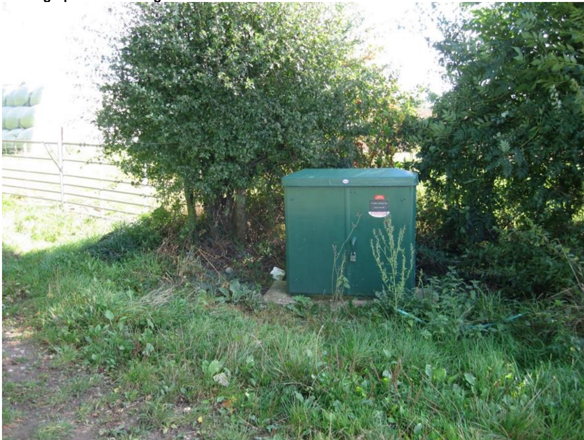
Photograph 4.1: Existing CP transformer rectifier cabinet.
