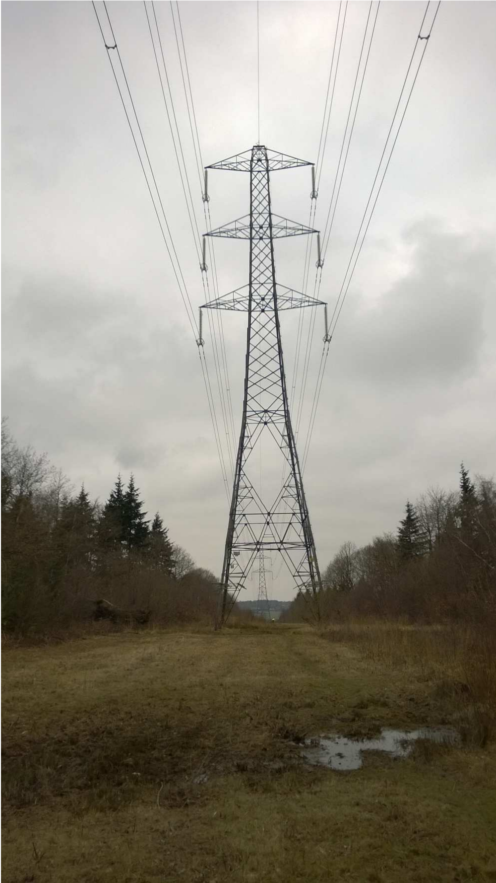
Fig 1: 400kV OHL passing through Clowes Wood looking south-east
