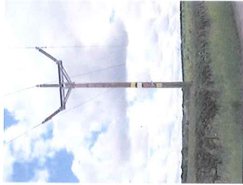
Trident single pole, 'trident' insulators
