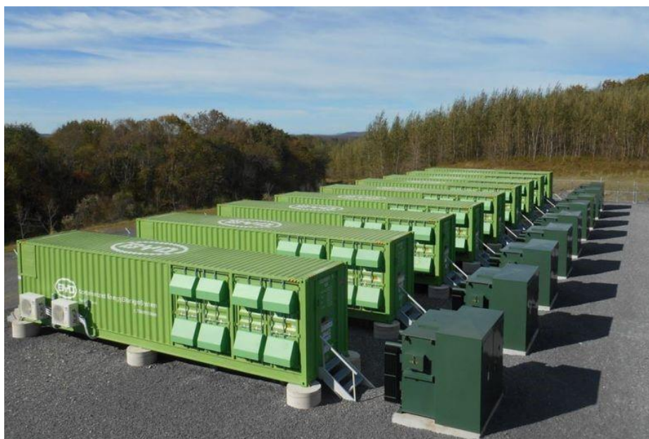
Image 3.4 – Example Battery Storage System Facility
