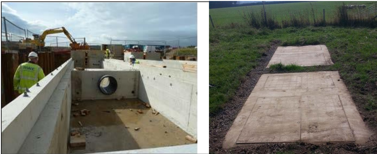
Figure 18: Typical Transition Joint Bay during construction (left) and two link boxes, each with manholes for electrical and optical cable joints, after reinstatement (right) (courtesy of RWE renewables UK Ltd).
