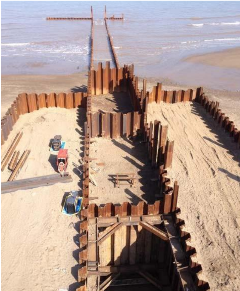
Figure 22: Example of an intertidal cofferdam installed using sheet piles. (courtesy of RWE renewables UK Ltd).
