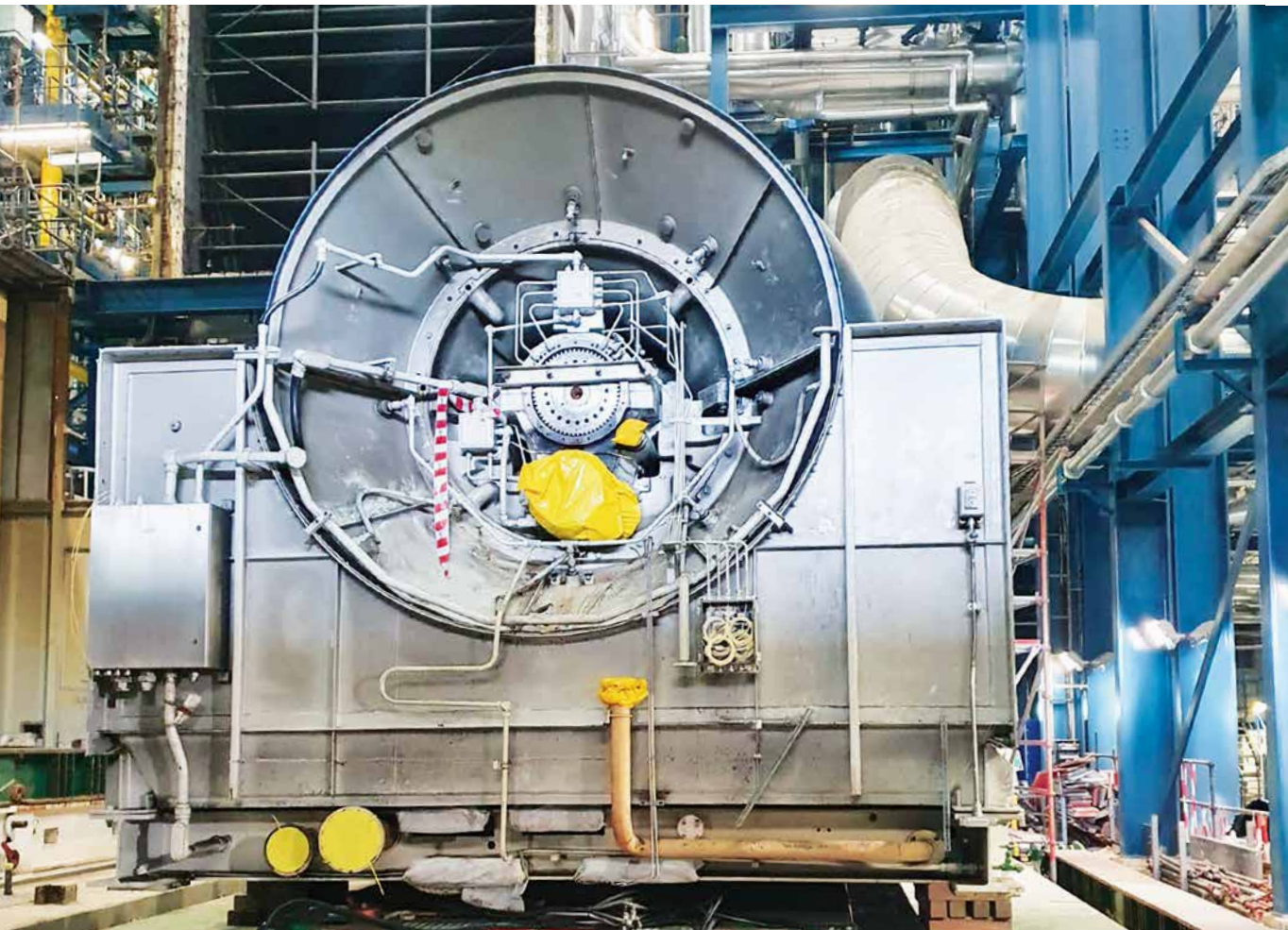
One of the two new gas turbo sets of the gas-and-steam turbine 2 during on-site installation.
