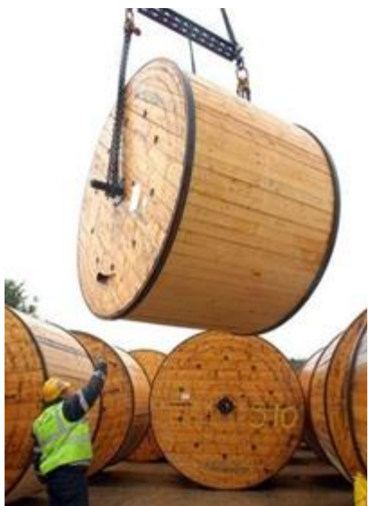
Figure 26: Example of a cable drum delivery to cable storage area (Courtesy of Scira Offshore Energy).
