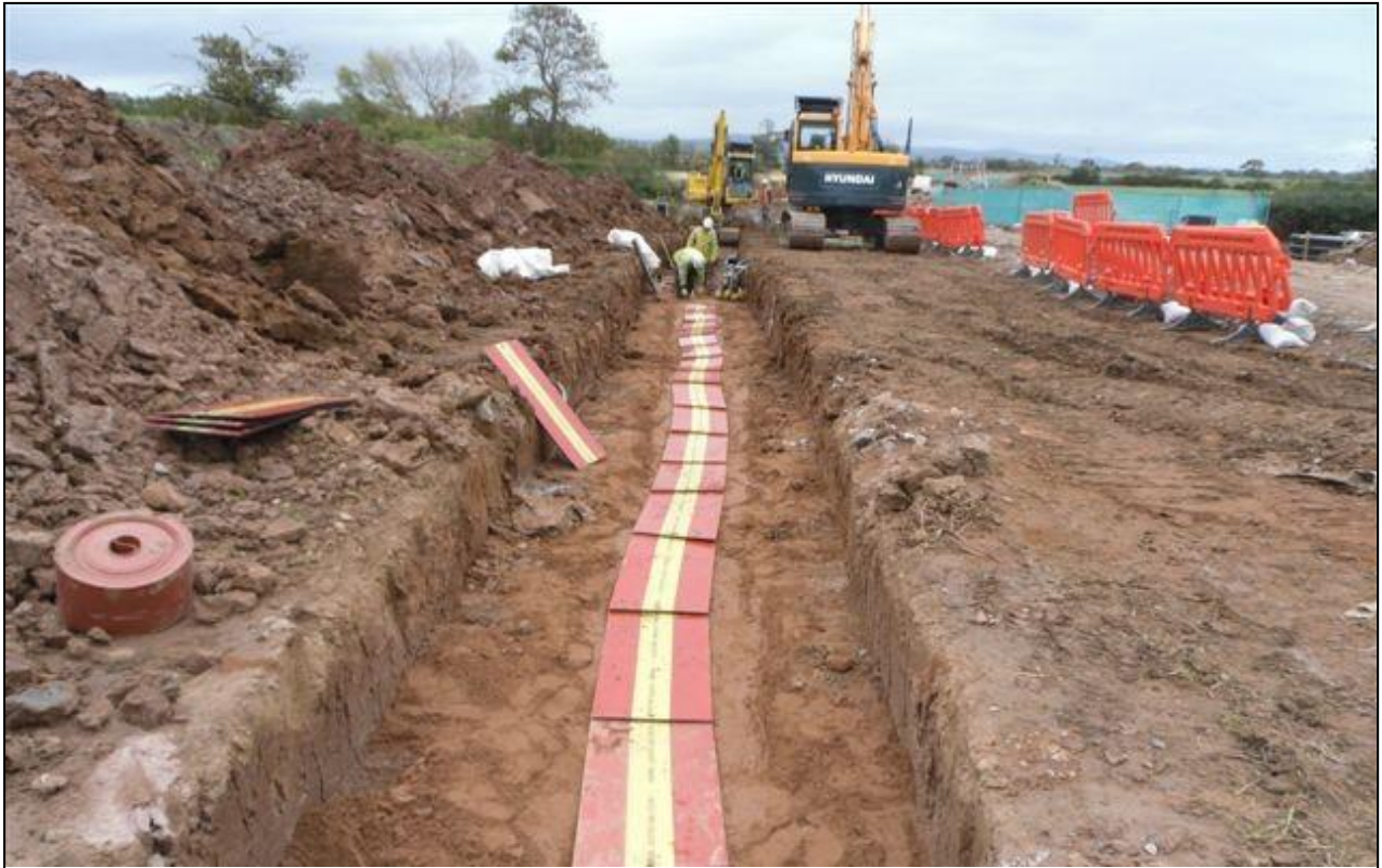
Figure 27: Cable trench having been partially backfilled, with cable marker boards (courtesy of RWE renewables UK Ltd).
