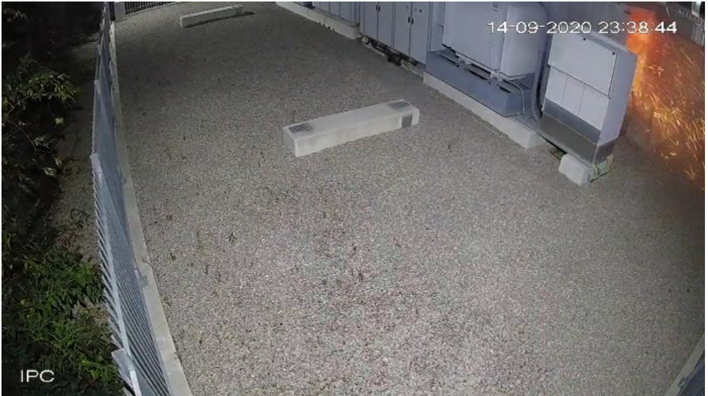
External CCTV showing flaming discharge consistent with a failing Lithium cell
