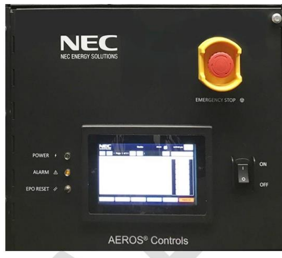
Image 7 is an example of the Control System Monitors at the Module, Rack, Zone, Powerblock and System Levels 6
