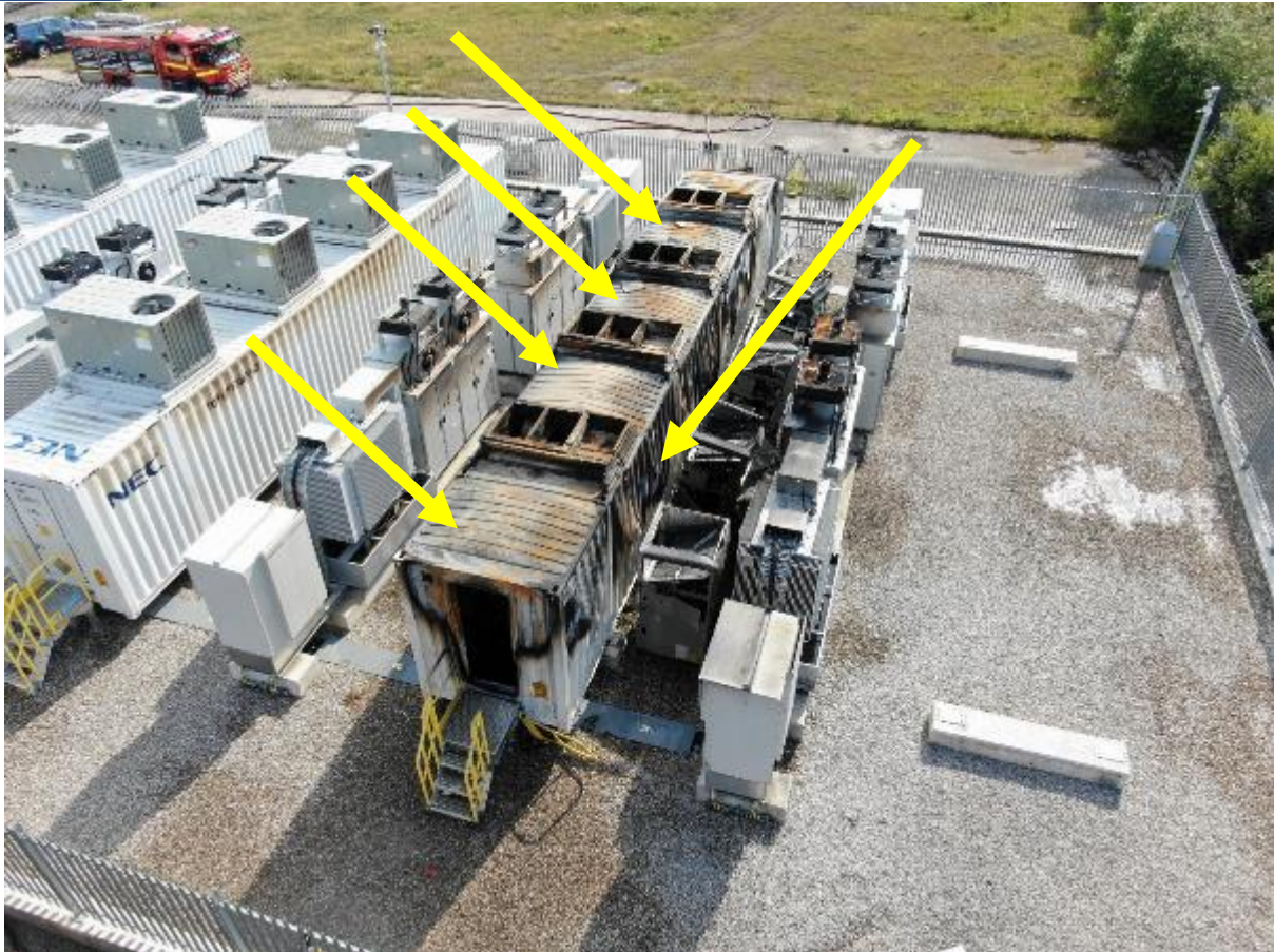
Image 2 shows the damaged container with signs of expansion/distortion that is equal across the container and not localised to the area of the initial failure.
