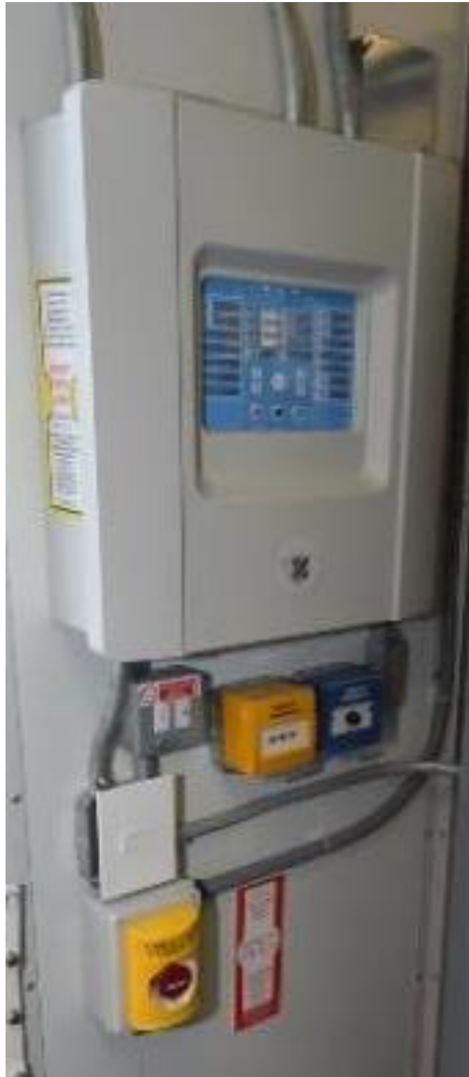
Alarm panel, emergency activation points and consumer unit
