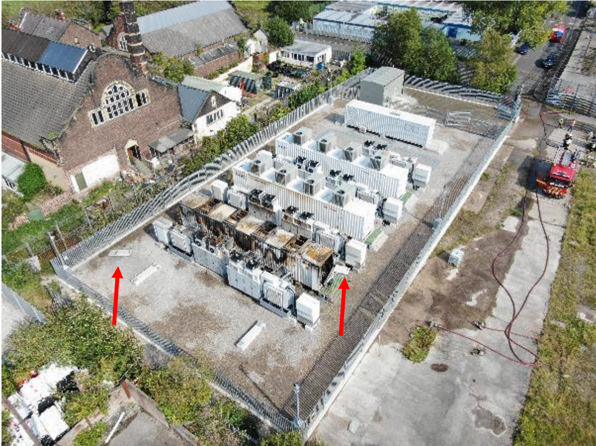
Air unit overview. The red arrows show the resting place of the doors
