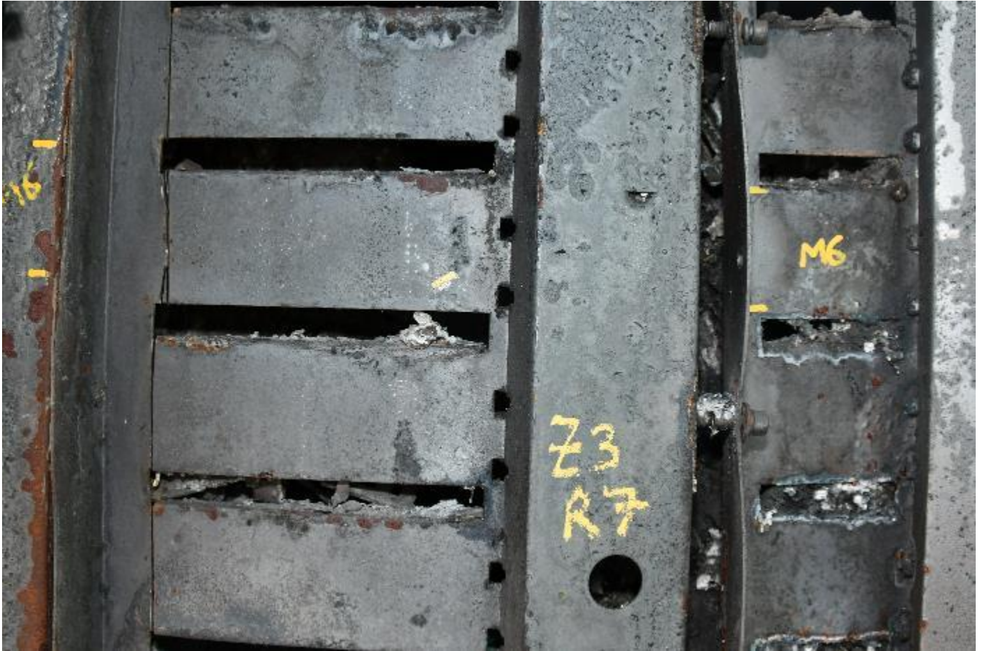
Image MB0_7397 shows where module 6 would have been pre fire. The modules had melted and collapsed.
