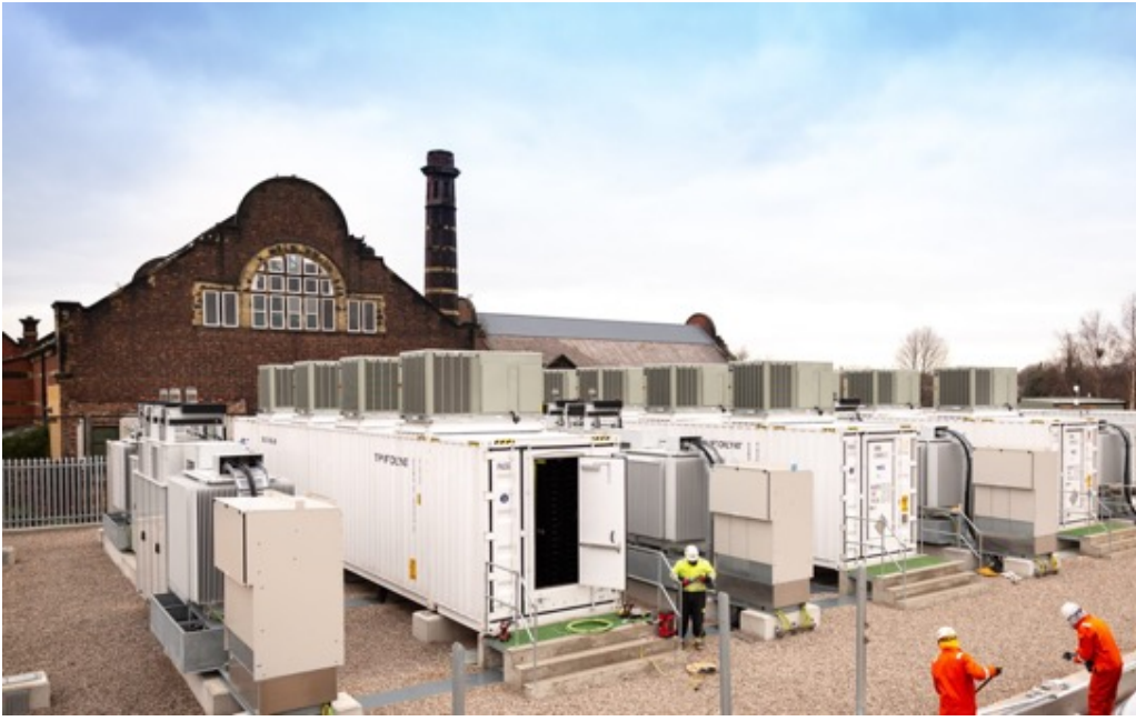
Figure 5: The 20 MWh BESS at Carnegie Rd, Liverpool. Courtesy Ørsted.
