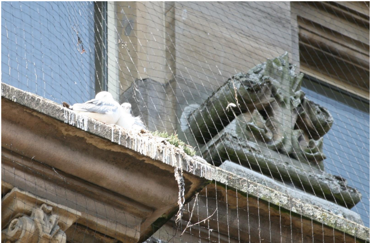
Photo 3.2.3. Kittiwake nest constructed on top of exclusion netting on a building at Newcastle Quayside.
