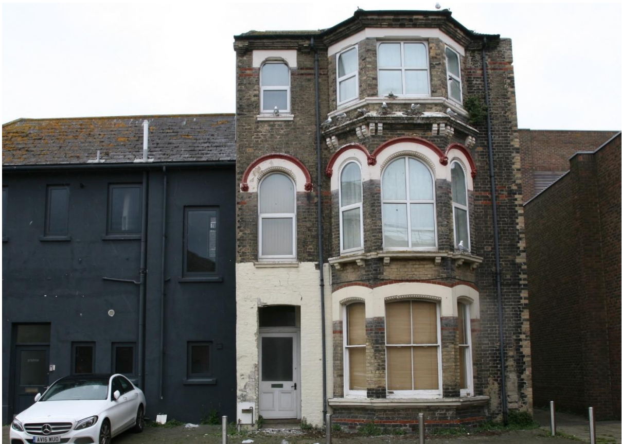
Photo E.12.1. Kittiwake nests on 2nd floor ledge and window ledges of house next door to Marina Theatre; May 2021.
