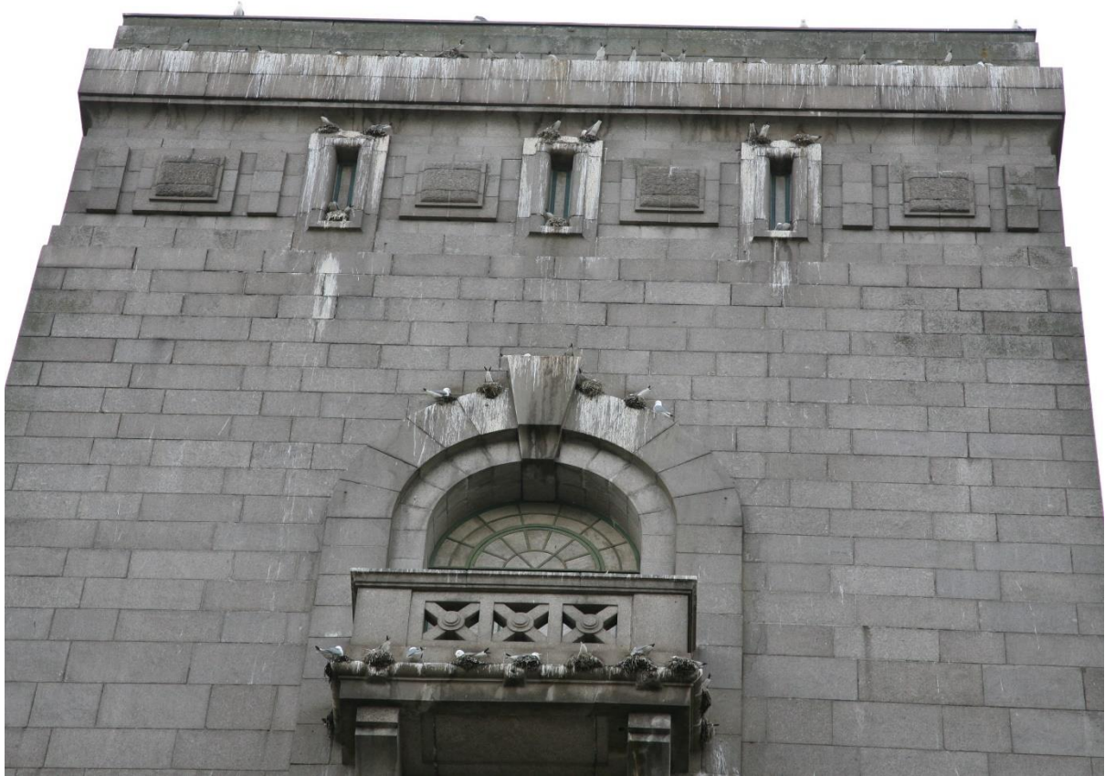
Photo D.16.3. Tynemouth Bridge. Kittiwakes nesting in window ledge slits, on the ledge around the balcony, on the stonework above windows, and along the ledge just below the top of the abutment; May 2021.
