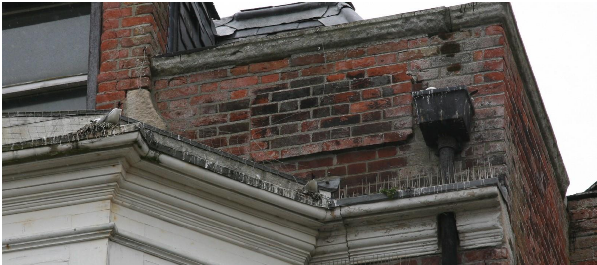
Photo E.17.5. Number 59 London Road North; May 2021.
