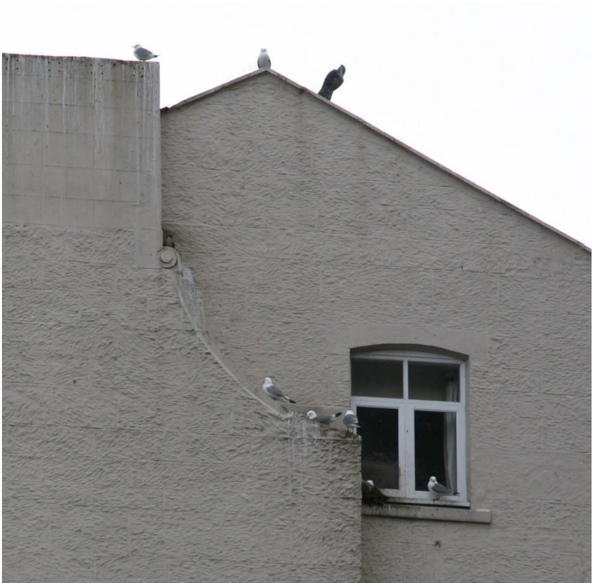
Photo D.15.2. Kittiwake nests on the end wall of Vermont Aparthotel, Newcastle Quayside; May 2021. The plastic falcon did not scare kittiwakes!
