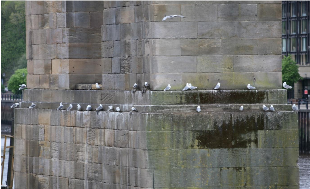
Photo D.14.1. One of the pillars of the High Level Bridge with a few kittiwake nests and numerous occupied sites that do not have nests; May 2021.
