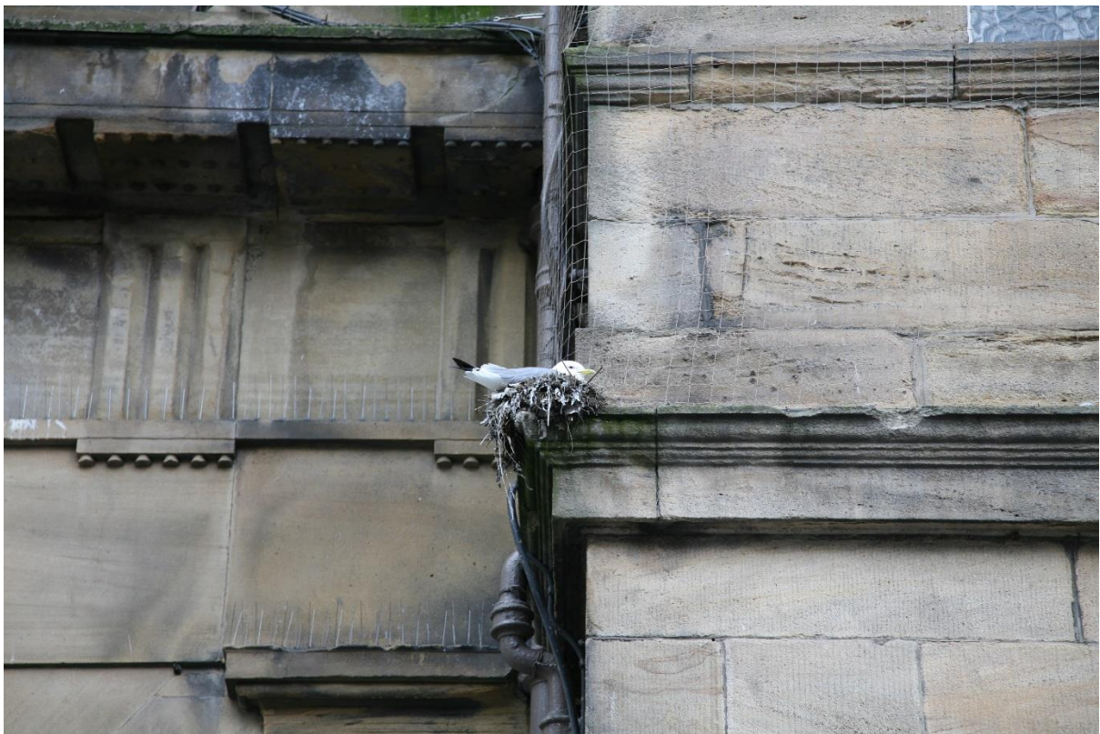
Photo D.5.1. Kittiwake nesting on top of exclusion netting on Guildhall (note also deployment of anti-bird spikes); May 2021. Most kittiwakes have been excluded from the walls of the Guildhall, and have moved onto the clock tower where they are not excluded (Photo D.5.2).
