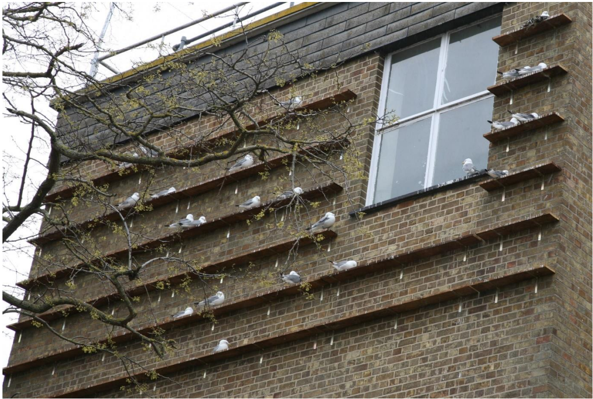
Photo E.15.5. Artificial ledges put up on the BT building in early May 2021, showing some occupancy by kittiwakes by late May (Photo taken on 26 May 2021), but little nest building by that date (unlike the nearly completed nests at most other sites).
