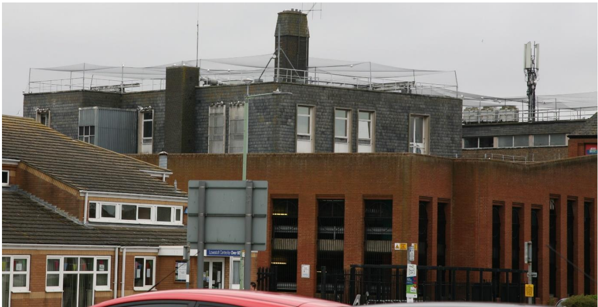
Photo E.15.2. BT building (the grey slate-tiled structure behind the red brick car park). Much of this building was fitted with exclusion netting early in 2021, but adverse publicity led BT to remove some of that netting in early May and to put up artificial ledges on one wall of the building to allow kittiwakes to relocate onto that area. Despite these actions, some kittiwakes managed to continue to use sites on window ledges and other ledges; May 2021.
