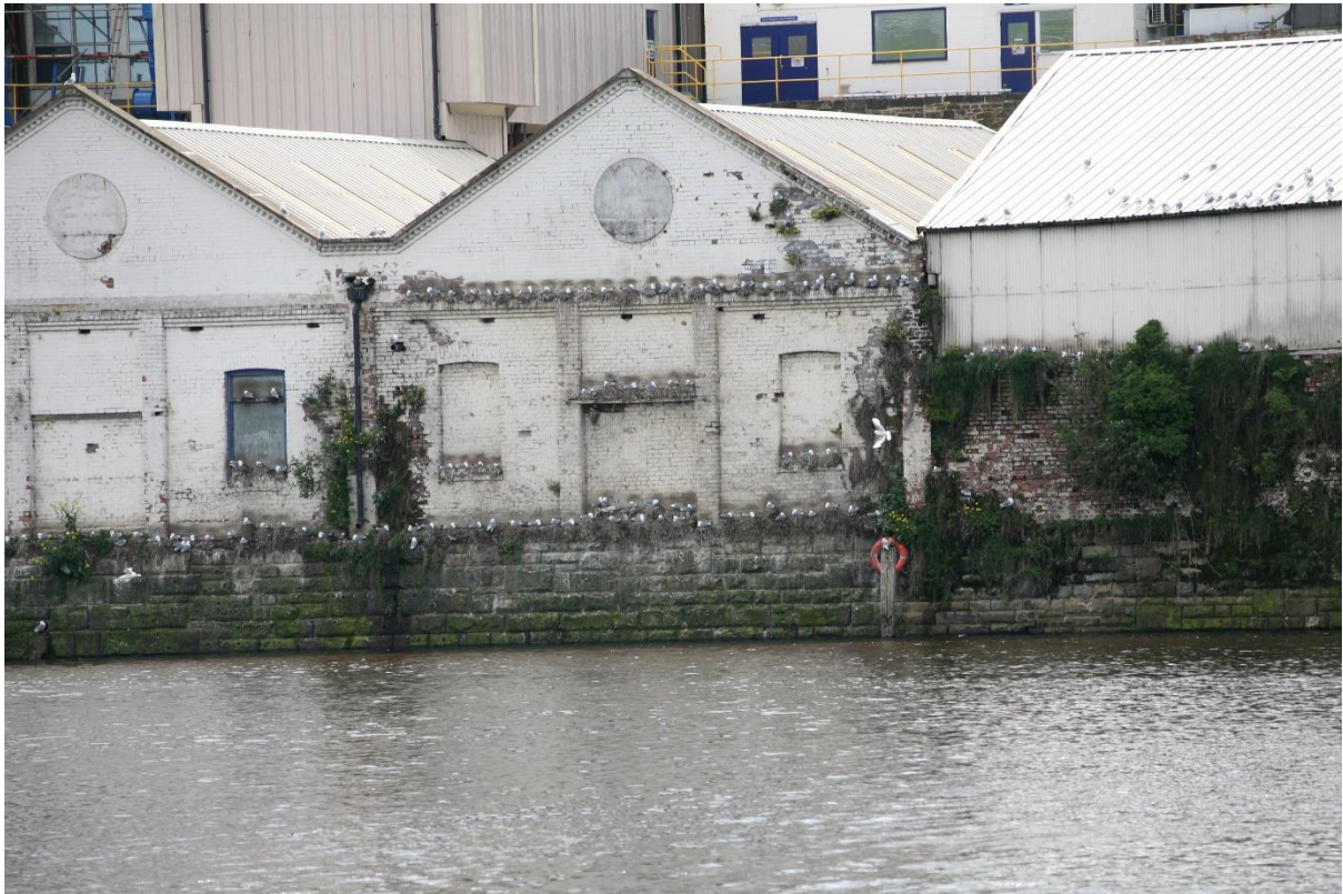
Photo D.2.1. Akzo Nobel, showing rows of kittiwake nests on narrow ledges on the north-facing side of the industrial buildings immediately on the south bank of the River Tyne; May 2021.
