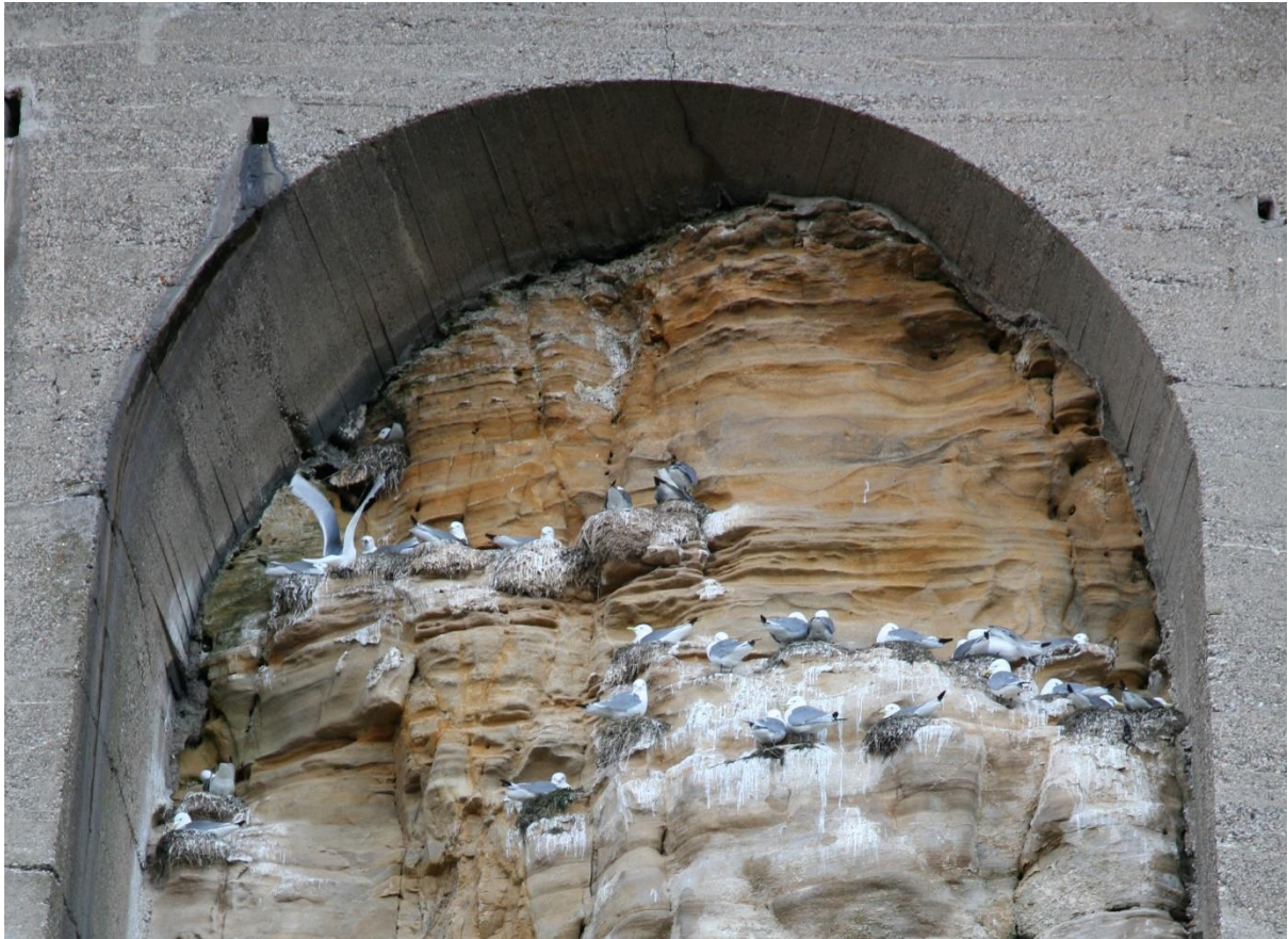
Photo D.1.3. Tynemouth, showing an example of kittiwakes nesting on the natural rock face but under the concrete arch of erosion defence; May 2021.
