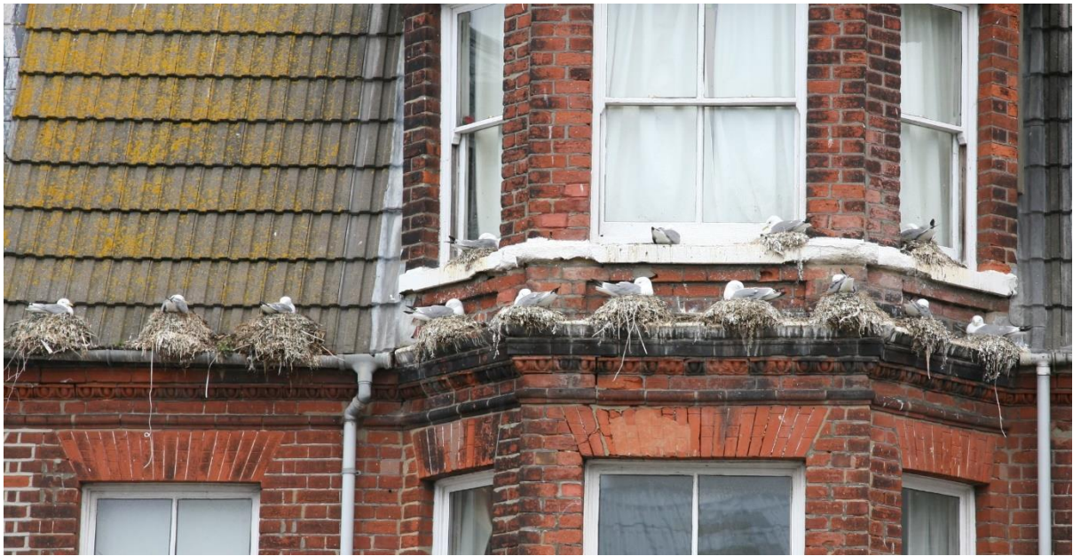
Photo E.9.3. Upper floor of 3 Battery Green Road; May 2021.
