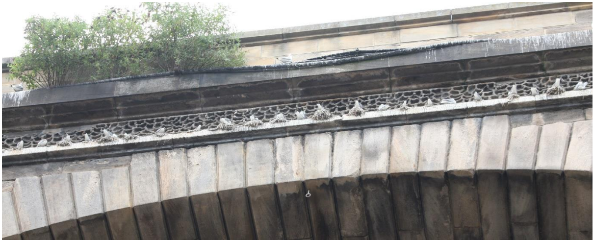
Photo D.11.1. Part of Dean Street railway bridge occupied by nesting kittiwakes all along the ledge; May 2021.
