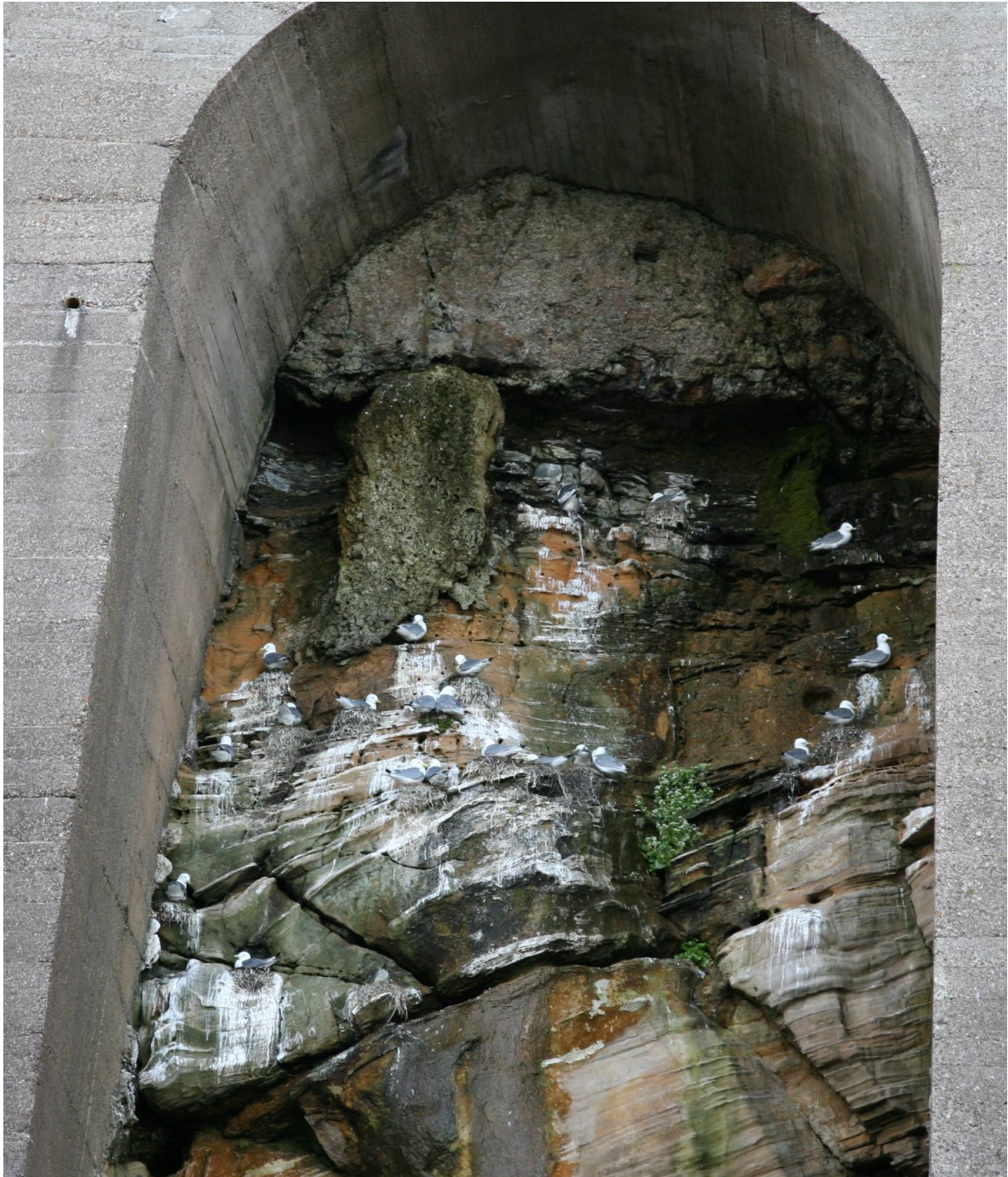
Photo D.1.4. Tynemouth, showing another example of kittiwakes nesting on the natural rock face but under the concrete arch of erosion defence. Note in this case much water seepage from the cliff that could affect nests; May 2021.
