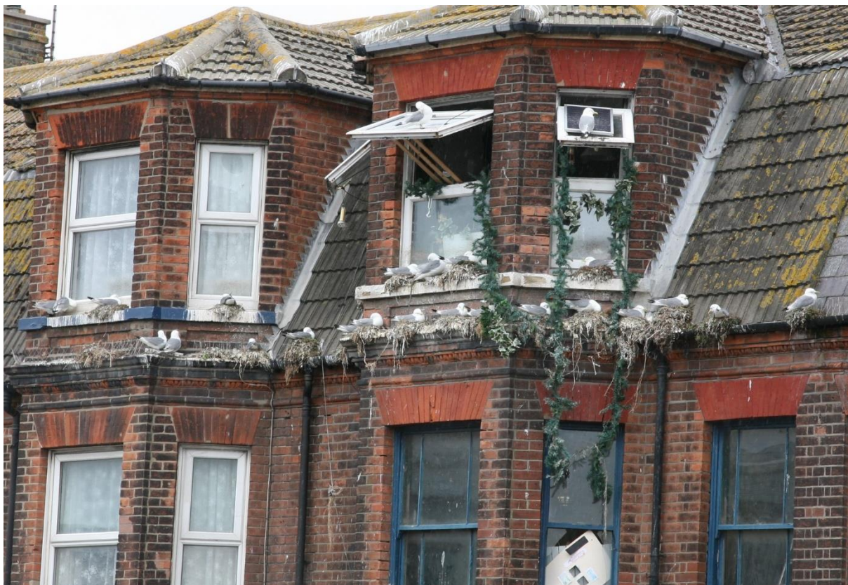
Photo E.9.2. Upper floor of 9 Battery Green Road; May 2021.
