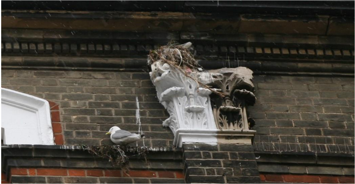
Photo E.17.1. Kittiwake nests on 41 London Road North (above Subway); May 2021.
