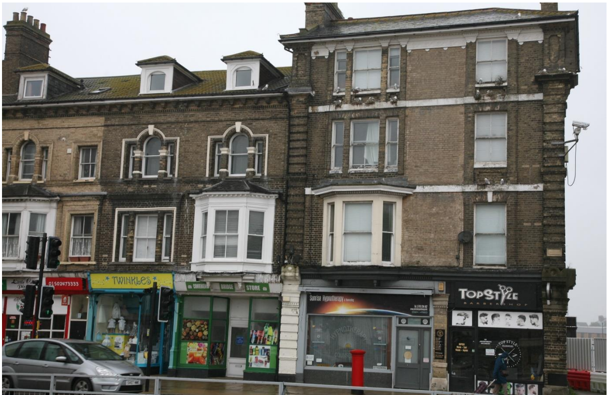
Photo E.18.1. Pier Terrace, with kittiwakes nesting on the end of terrace building; June 2021.
