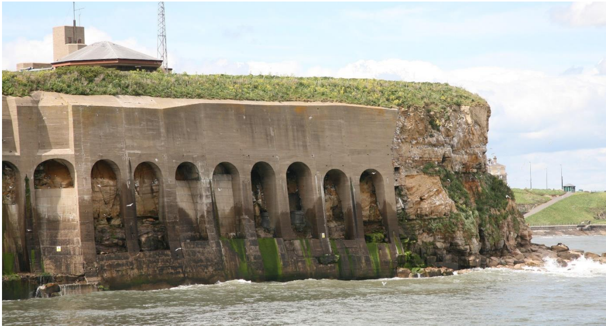
Photo D.1.1. Tynemouth, from the south-east, showing part of the natural cliff and the part buttressed with concrete erosion defence arches; kittiwakes nest on the natural cliff and under the concrete arches; May 2021.
