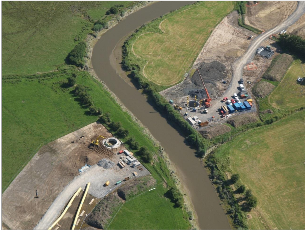
Plate 5.21 Aerial image of example trenchless river crossing with stop end (Source: Courtesy of J Murphy & Sons Ltd)
