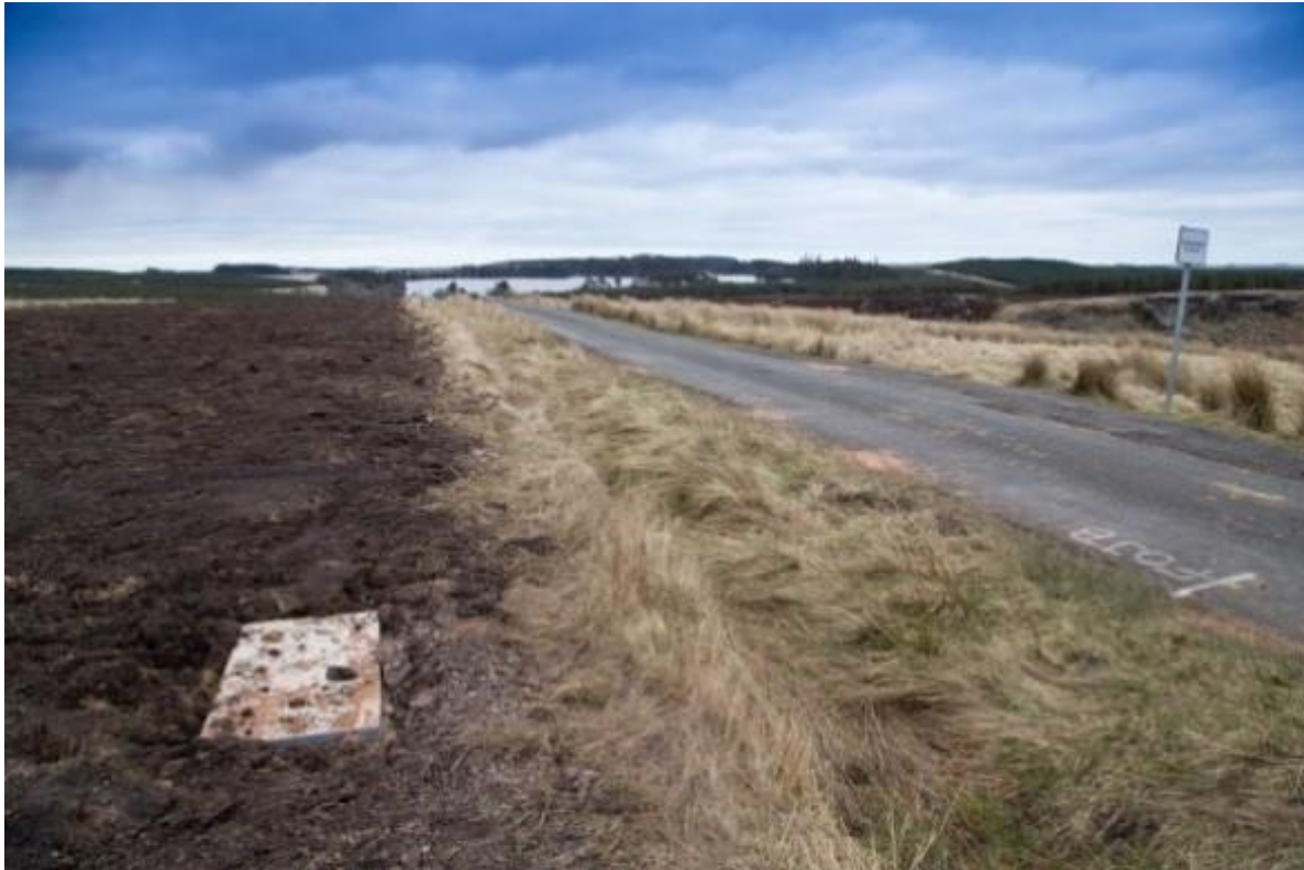
Plate 5.14 Example below ground link box following reinstatement (Source: Ray Wind Farm, Vattenfall Wind Power Limited)
