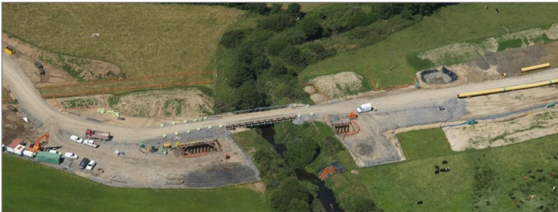
Plate 5.19 Aerial image of example trenchless river crossing with temporary bridge (Source: Courtesy of J Murphy & Sons Ltd)
