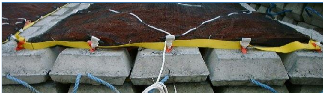
Plate 5.11 Frond concrete mattress (Source: www.pipeshield.com )
