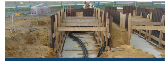
Transition joint bay. This is the onshore cable running up to the transition joint bay (concrete floor). The next step will be pulling the offshore cable into this location for the joint to be made. This arrangement is a concrete floor only design, with temporary shuttering to the sides. The alternative is a fully concreted box with concrete sides.
