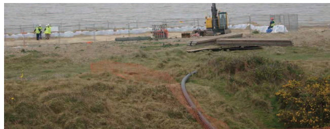
Horizontal directional drilling outfall. The image shows preparations on the beach to excavate the HDD exit.
