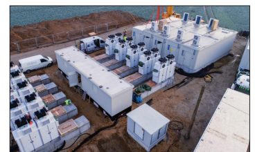
A typical lithium ion battery park and transformer complex
