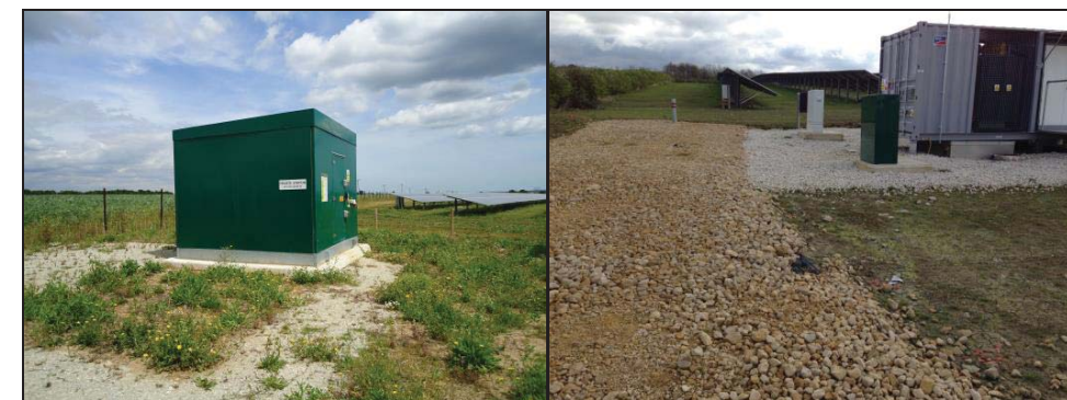
Plate 7: Typical ancillary structures on crushed stone at solar farms
