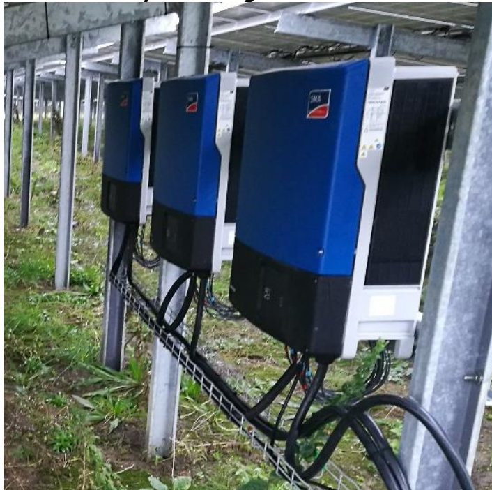
Plate 5.7 Example of string inverters mounted beneath solar PV modules
