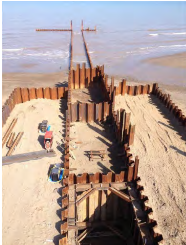
Figure 2-6: Illustration of sheet piling used for intertidal cofferdams (Sheet Piling UK Ltd).
