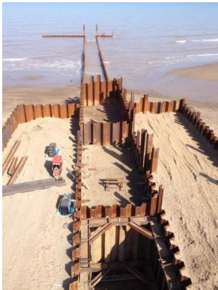
Figure 2.7: Illustration of sheet piling used for intertidal cofferdams (Sheet Piling UK Ltd).
