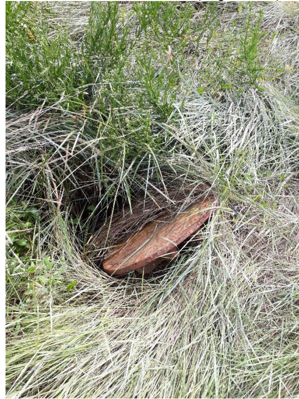
Photo 15: Close up photograph of the tidally flapped outfall (wedged open at the time of this photo) in the grass below the rock armor sea defence for the Cliffsend landfill (August 2017).
