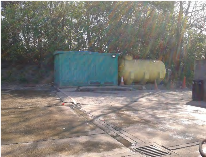
Picture 2 Above ground tank used as part of the car wash facility
