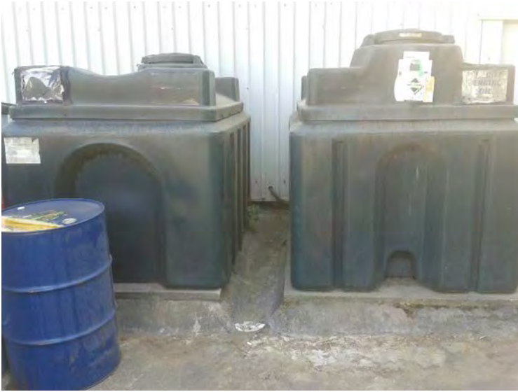
Picture 18 New oil and fuel storage tanks
