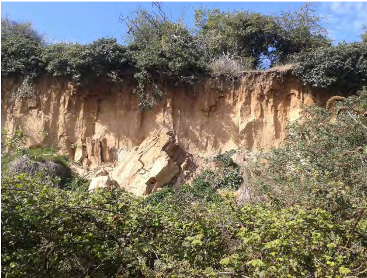
Picture 26 View of cliffs behind Pegwell Bay Hoverport, note apparent instability of cliff
