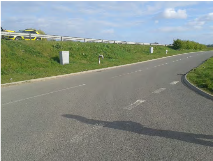
Picture 15 Breather pipes at the entrance of Weatherlees WWTW
