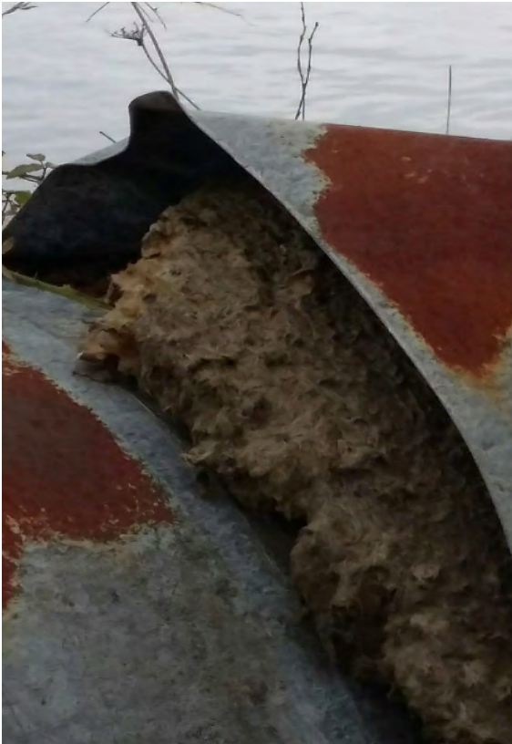
Picture 6 Pipeline lagging
