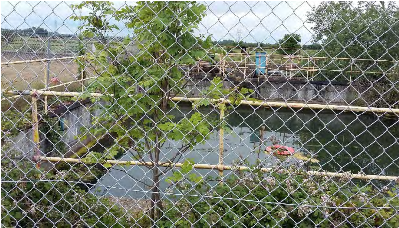
Picture 14 WWTW on-site at the former Richborough Power Station
