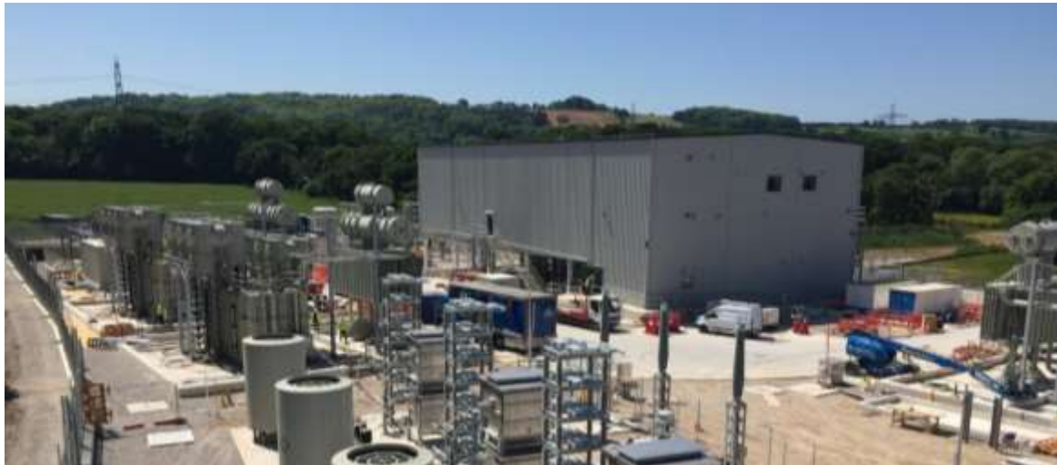
Figure 4.1: Walney Extension Onshore Substation as constructed
