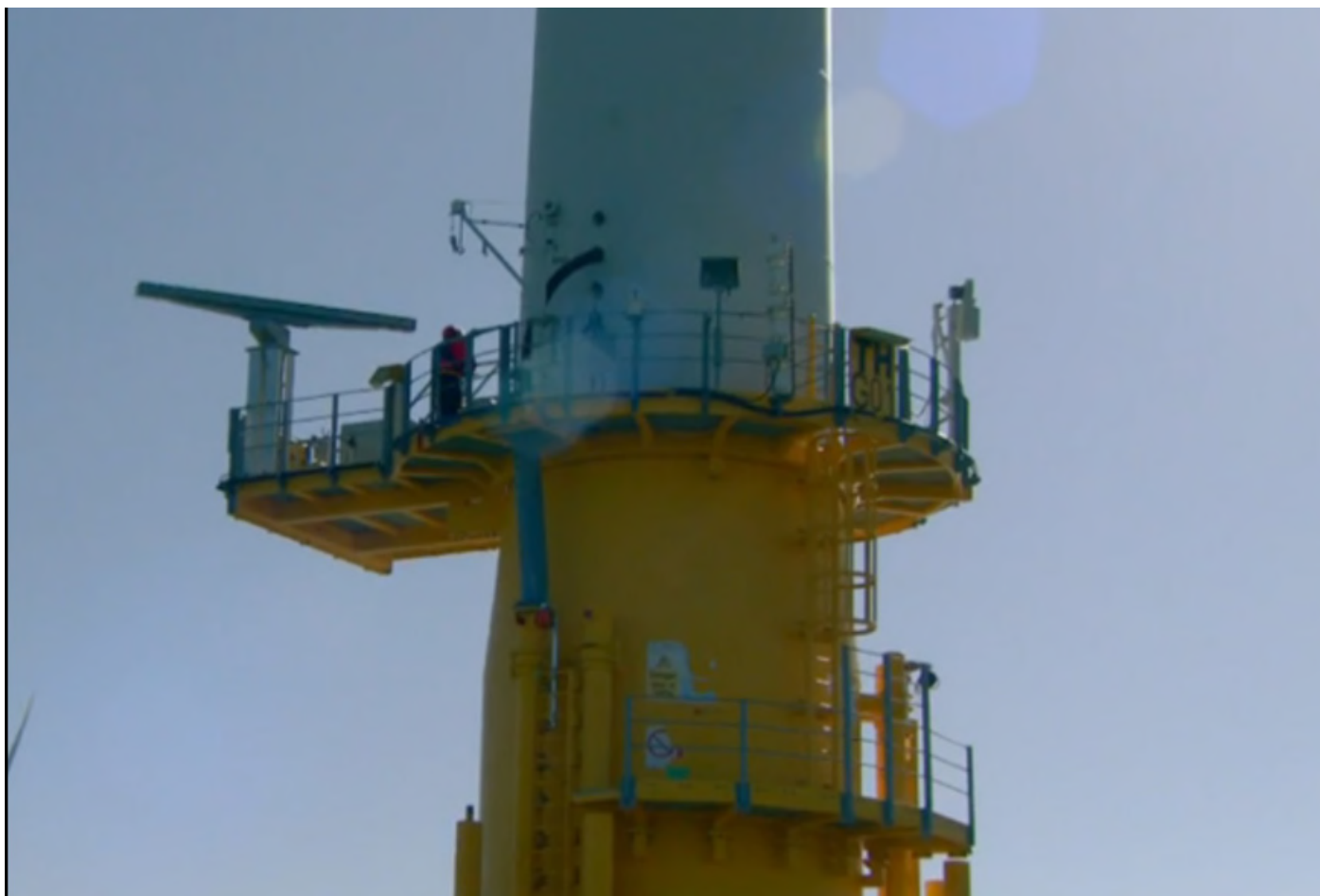
Figure 1. SCANTER 5000 radar installed on the laydown area of the work platform of turbine G01 at Thanet Offshore Wind Farm.
