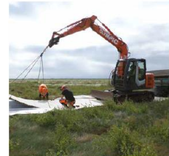
Setting up the ground conditions on the salt marsh for Race Bank Offshore Wind Farm.
