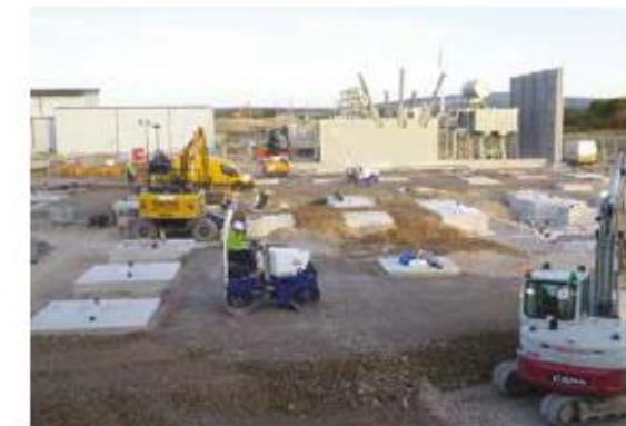
Typical vehicles during the construction of the substation at Walney Extension Offshore Wind Farm.
