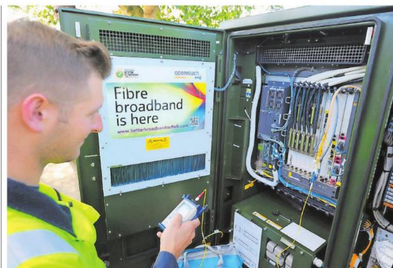
A field technician looking at a roadside cabinet.
