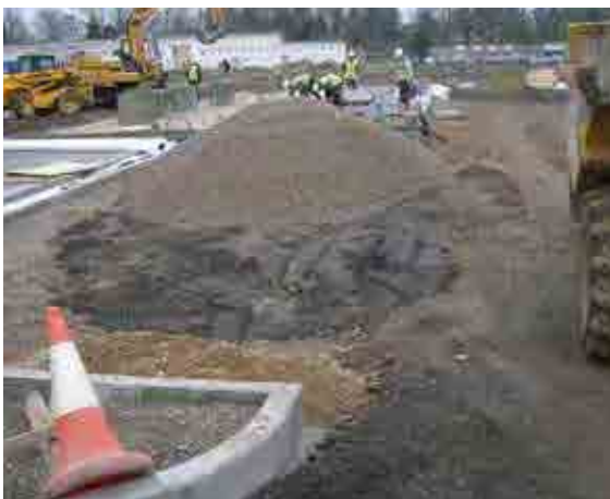
Figure 31.1 Inadvertent compaction of subgrade below pervious surface construction intended to infiltrate water to ground. Compaction will reduce the infiltration rate (courtesy EPG Limited)
