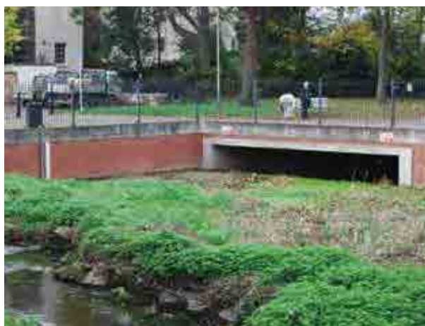
Figure 28.11 Example of landscaped flow splitter structure, River Chelt (courtesy Illman Young)
