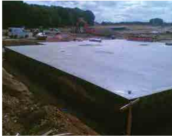
Figure 21.3 Frame covered by outer skin (geomembrane in this case) (courtesy EPG Limited)
