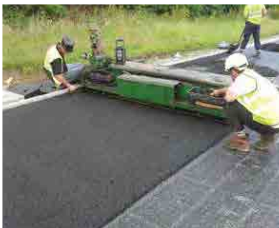
Figure 20.10 Construction of sports drainage and attenuation layer below school sports pitch in Hull (courtesy Phil Tomlinson)
