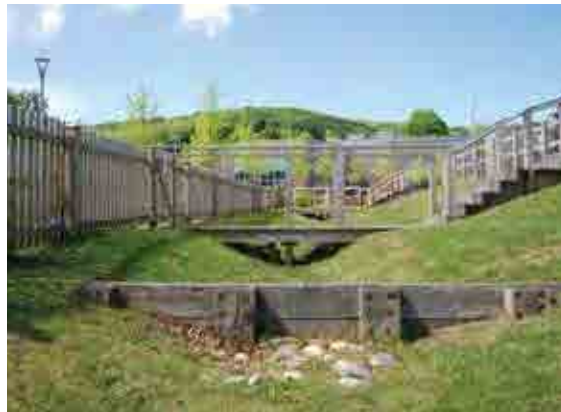
Figure 17.15 Timber check dams, Rednock School, Gloucestershire (courtesy Illman Young)
