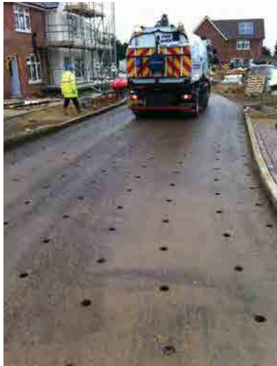
Figure 20.29 Layer of protective DBM over sub-base after coring and before laying concrete block permeable paving (courtesy Peterborough City Council)
