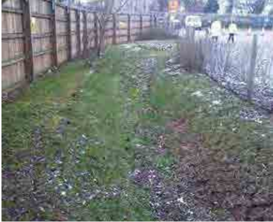
Figure 30.6 Example of topsoil retention on slope using cellular confinement (courtesy EPG Limited)
