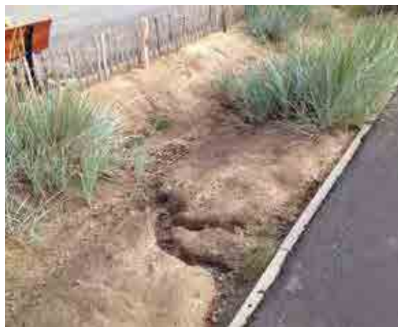
Figure 31.2 Absence of erosion protection before establishment of vegetation (courtesy EPG Limited)
