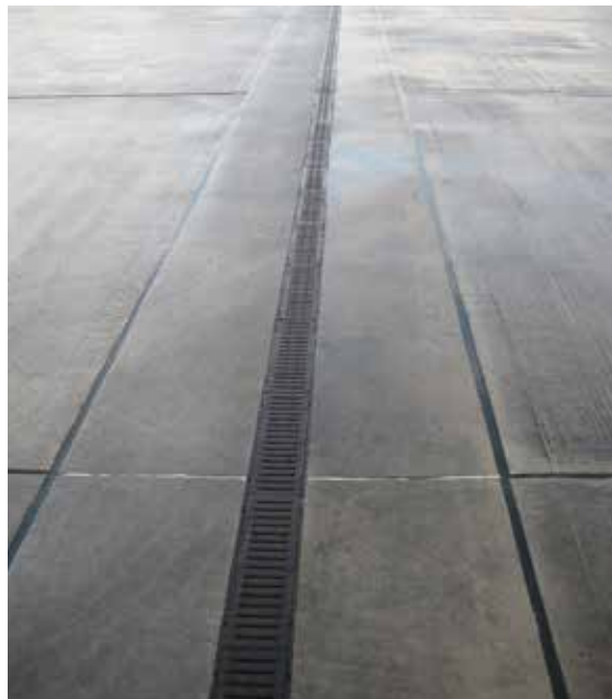
Figure 20.9 Macro pervious pavement in warehouse yard in north-west England with channel collection/pollution trap and concrete pavement construction (courtesy EPG Limited)
