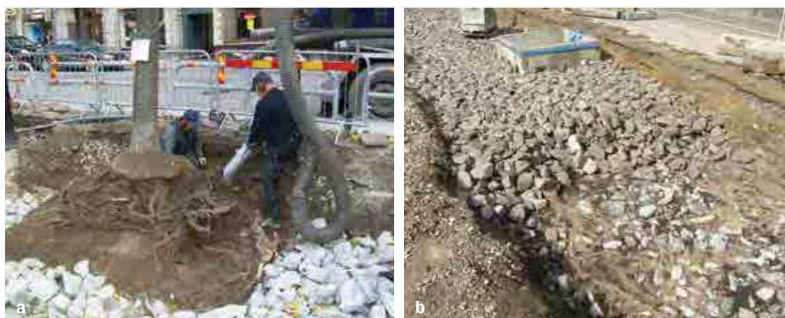
Figure 19.7 The use of structural growing media in retrofitting (a) and new-build (b) (courtesy Björn Embrén)
