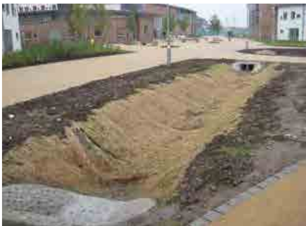
Figure 17.16 Swale during construction showing coir matting used to protect soils from erosion before the establishment of vegetation, University of York (courtesy Arup)
