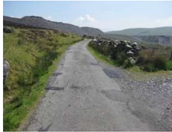
58. The quarry access road is of mixed condition throughout. There are existing signs of cracking and there is no kerblines just a grass verge. Remains from previous quarry activity feature to the left of the highway.
